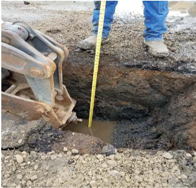
Photograph 3: Taken facing North East. Western pothole. No UST was found at in this pothole.
