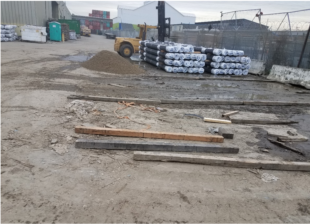
Photograph 1: Taken Facing North East. GPR anomalies detected in this area, indicating the possible presence of a UST.
