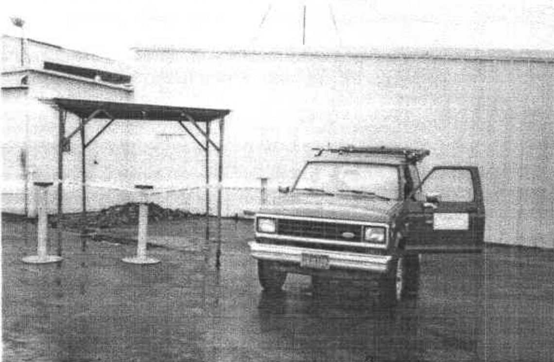
Picture 4: Cleaned the area and placed a barrier around the excavation. June 29, 1992
