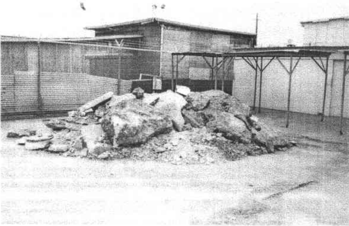
Picture 11: Pile of concrete and asphalt. Previously used as a surfacing material above the excavation. August 3, 1992
