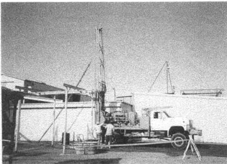
Picture 9: November 3, 1992 Drilling rig at location of pilot boring PB-MW3 and monitoring well 9MW3.
