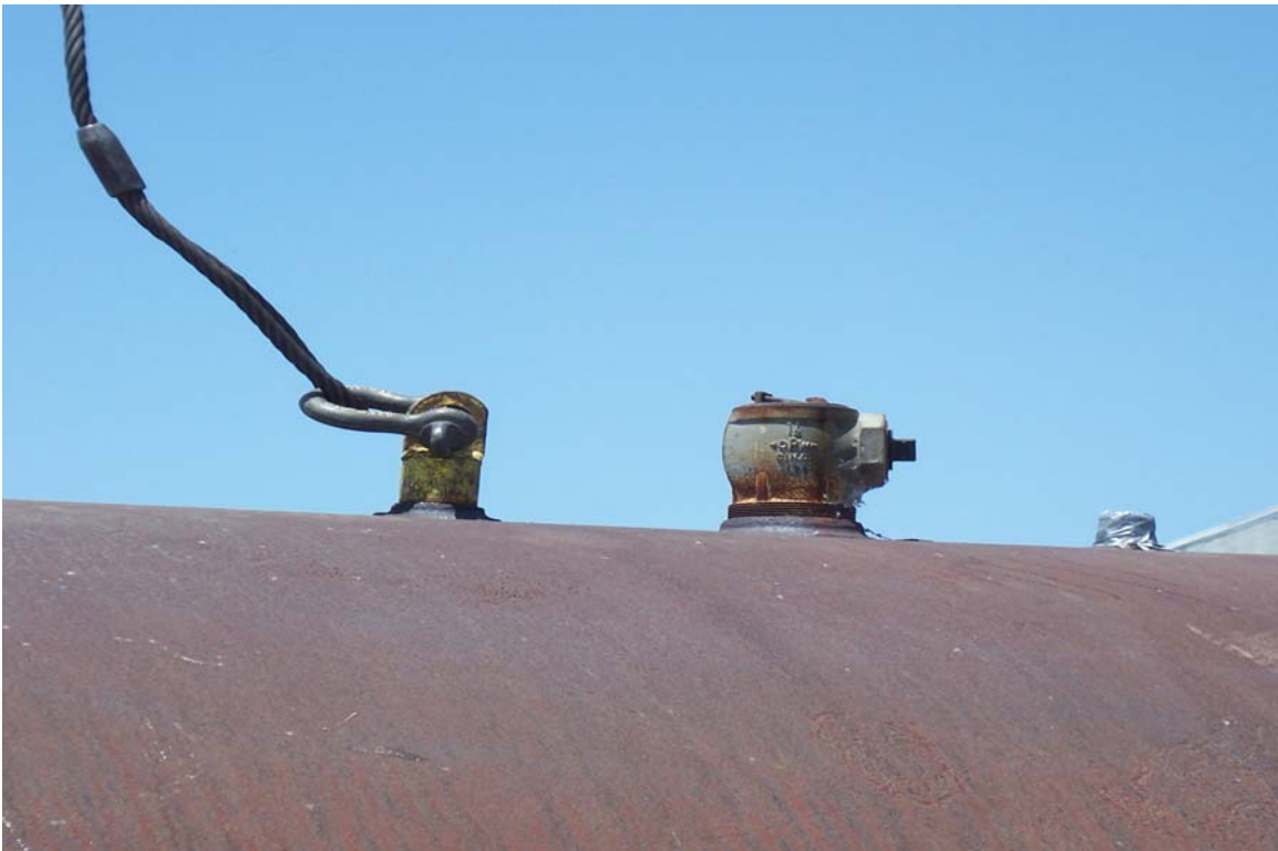
8. View of OPW brand ball and cage float overfill prevention device attached to AST T-2.
