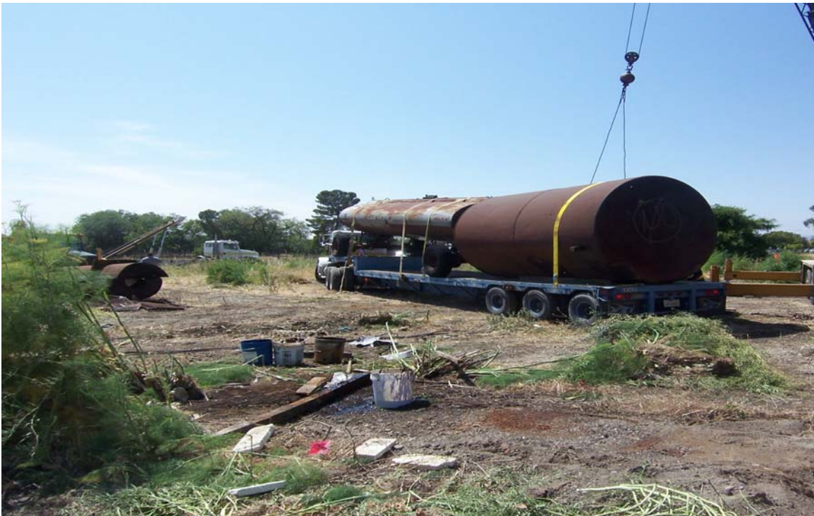
10. AST T-2 loaded onto the ECI truck after the sludge had finished draining, the hole in the tank had been plugged with wood, and the tank had been cleaned off in the vicinity of the leak. The former location of AST T-2 is shown in the foreground. The former location of AST T-1 is on the right behind the buckets.
