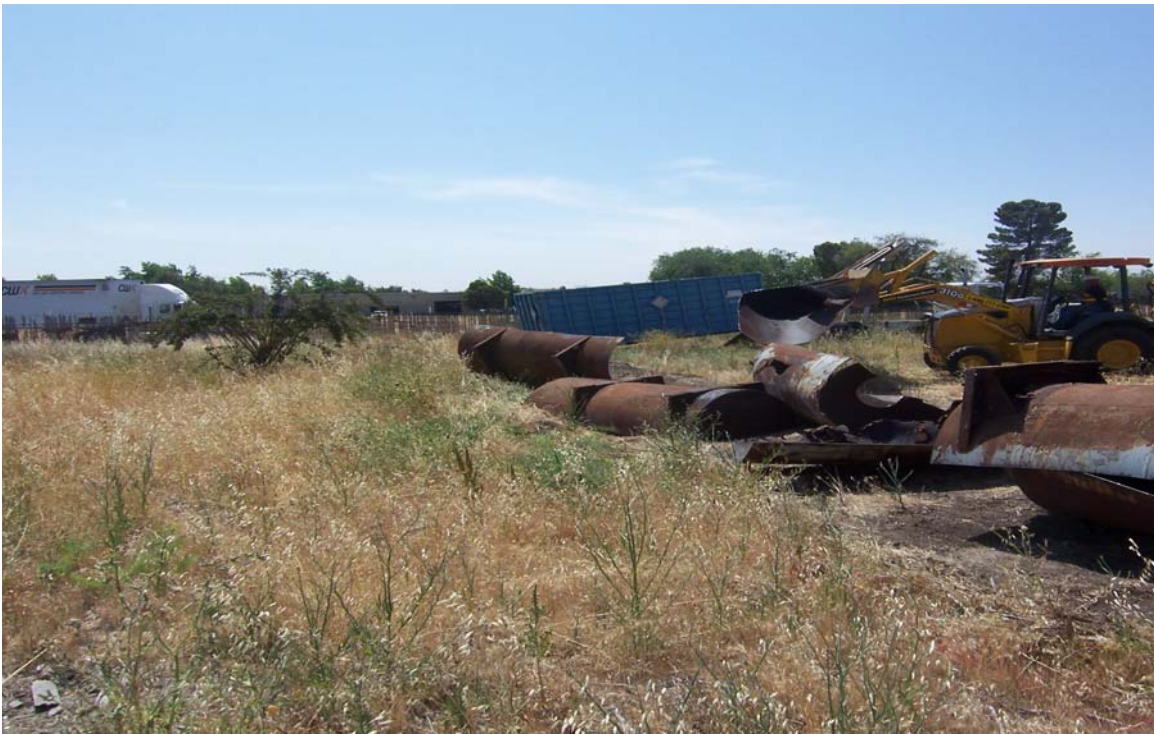
6. Former AST T-1 after being cut into pieces to be hauled offsite as non-RCRA hazardous waste. The scraps are being loaded into the roll-off bin in the background.
