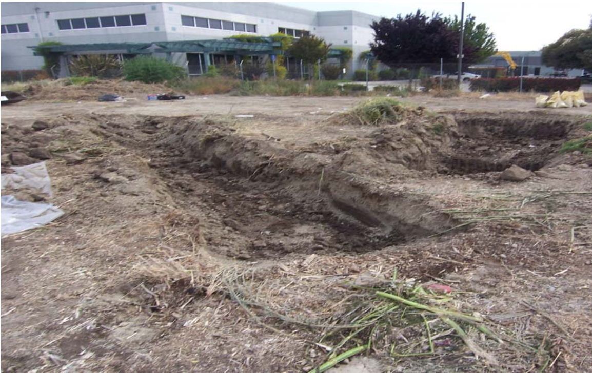
18. Excavations in the former locations of AST T-1 (left) and AST T-2 (right).
