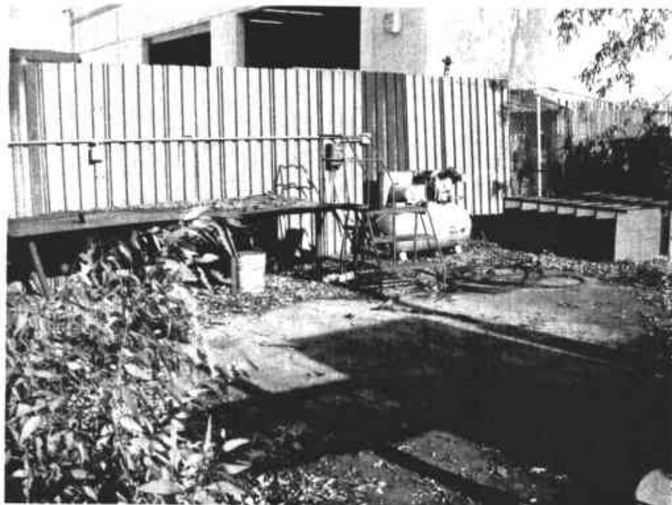
Photo no. 5: The area on the north side of the property where an underground tank was removed.
