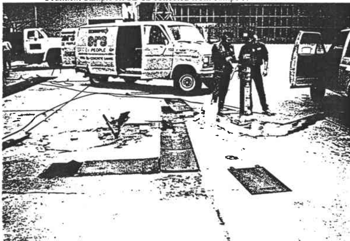
Borehole Samples H9S-05 and H9S-06 collected on eastern and western side of former hydraulic lift
