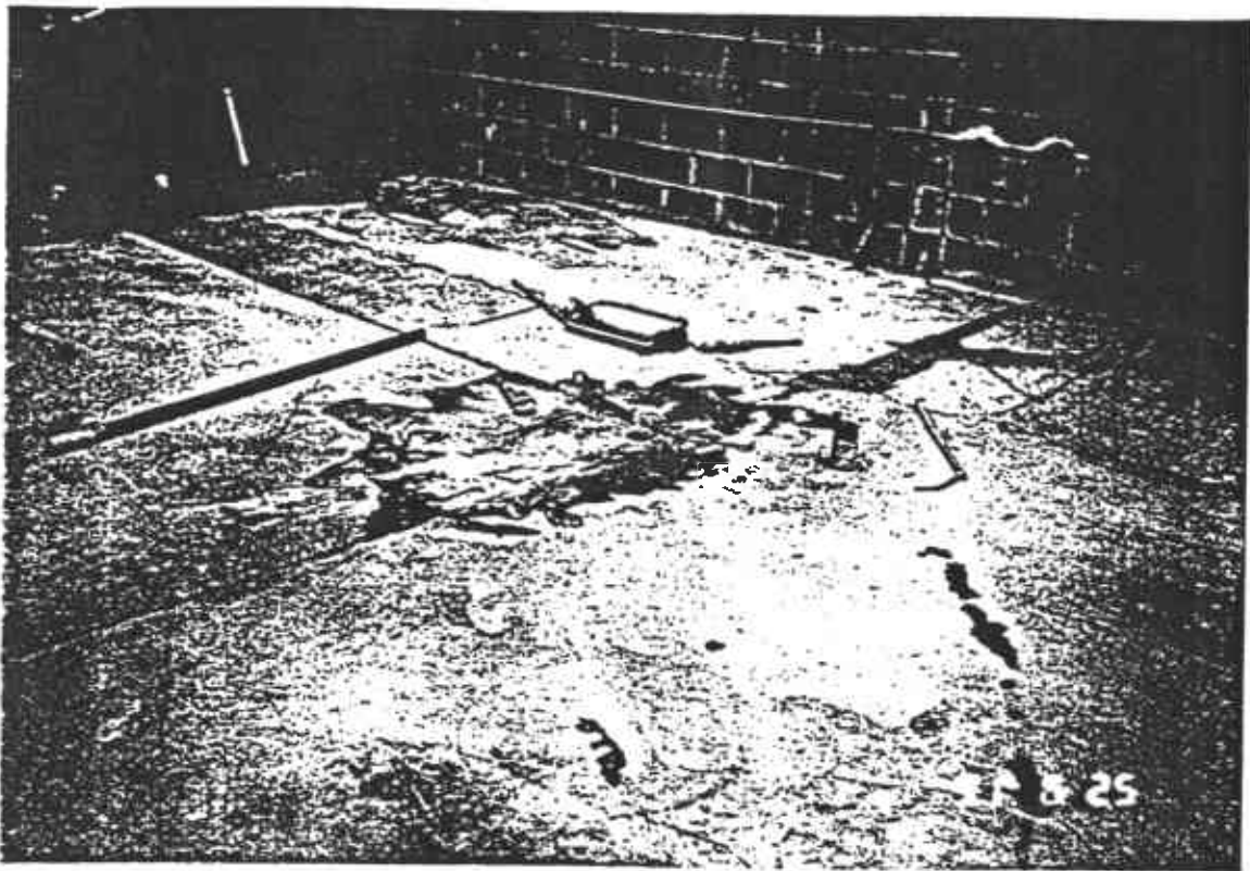
Borehole Sample H9S-13 and H9S-14 collected outside the southeast corner of Hangar 9 in the former drum storage area
