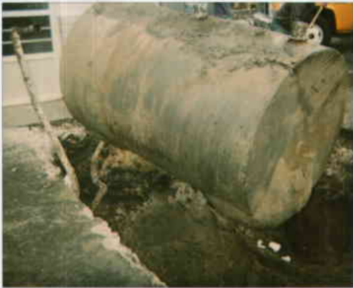
WASTE OIL TANK
