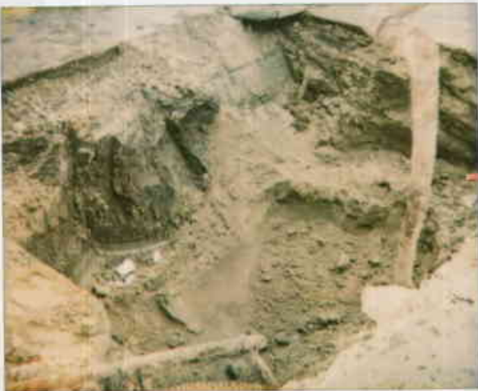
WASTE OIL TANK PIT
