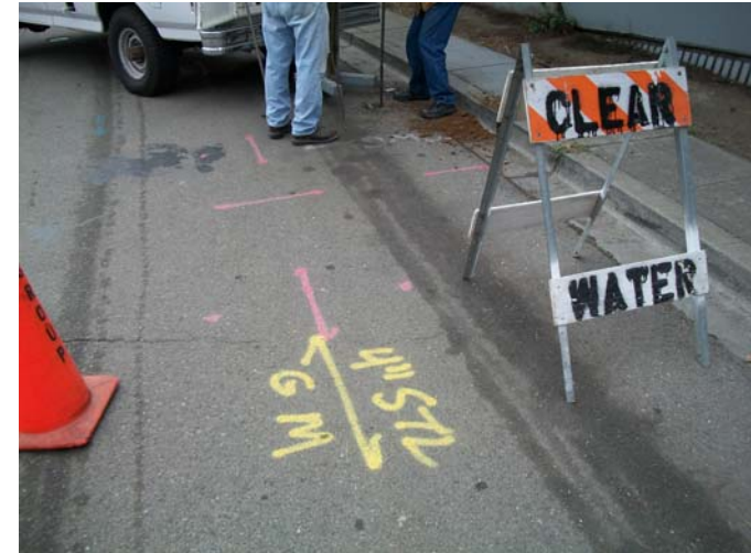
Hand auger S12 showing 4" gas line
