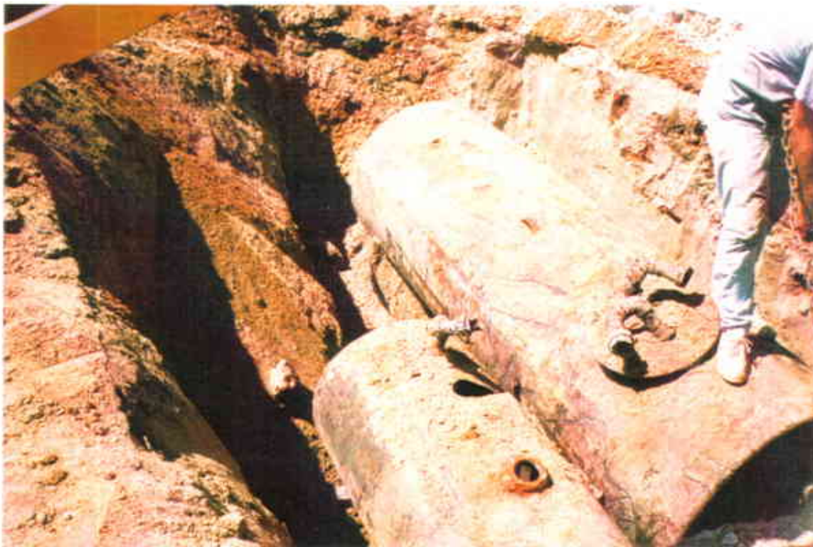
a. Tank Protect Personnel began excavating UST #10, waste oil tank and UST#11, lube oil tank.
