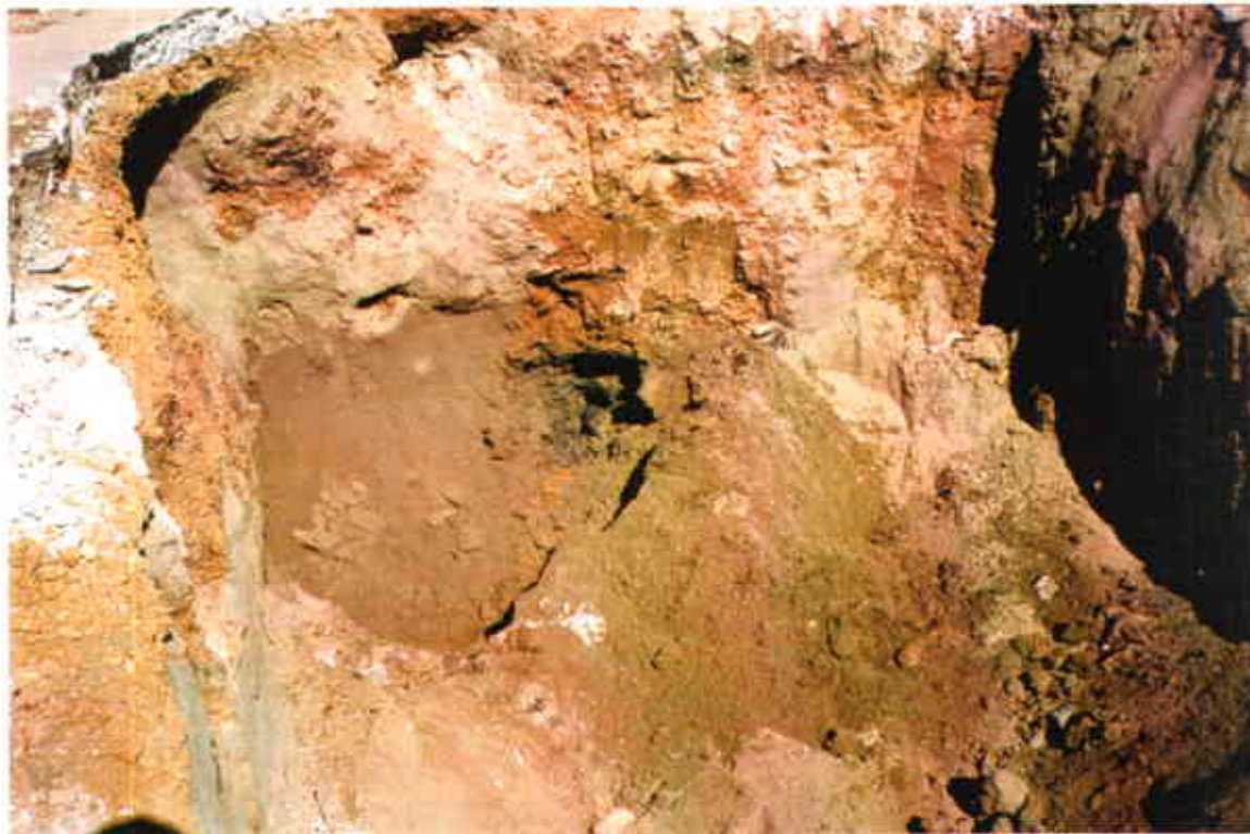
j. The removal of the USTs are completed. Soil samples were collected from a random location with the backhoe.
