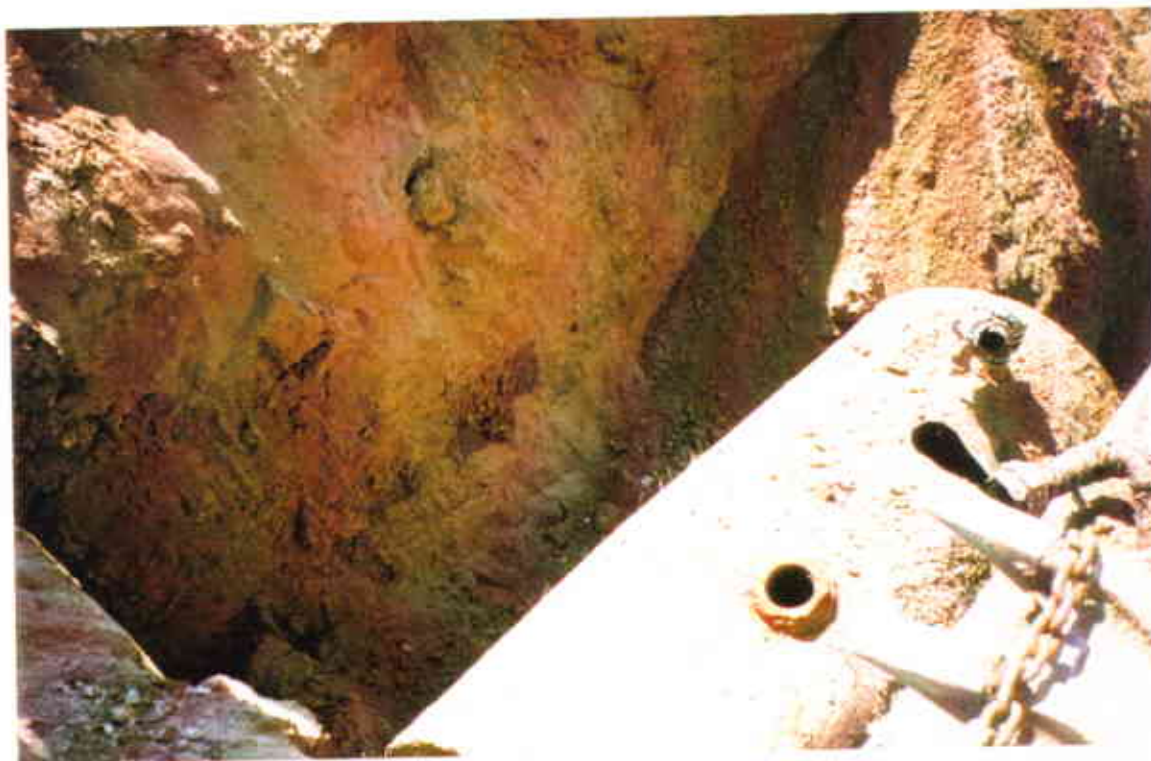
d. The atmospheres of the USTs are being inerted with carbon dioxide.
