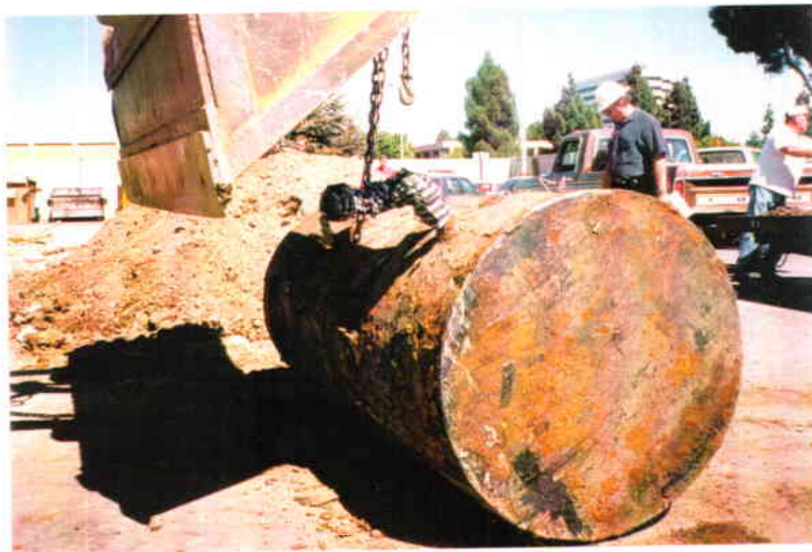
f. UST#11 was removed from the excavation area and staged for inspection by City and County Officials.
