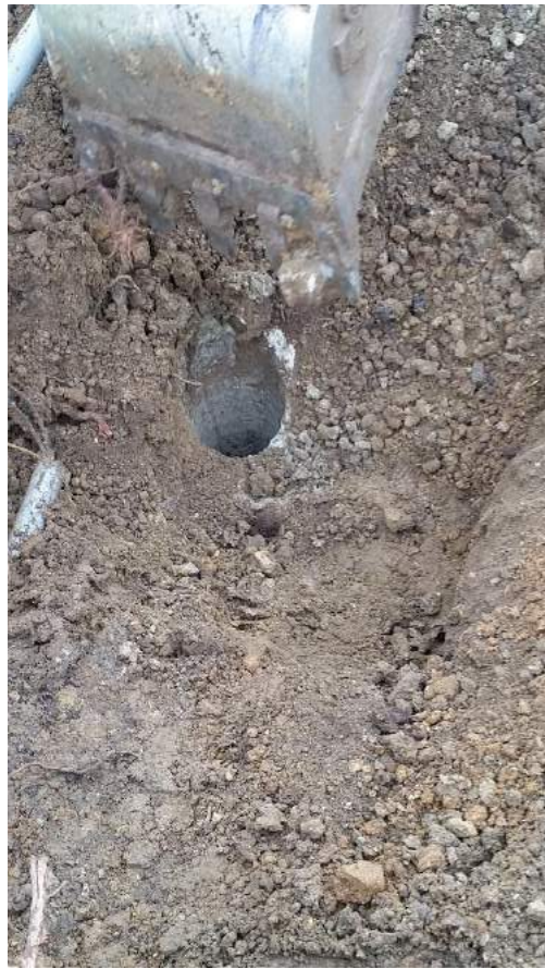
Figure 4: Storm Drain Damage
