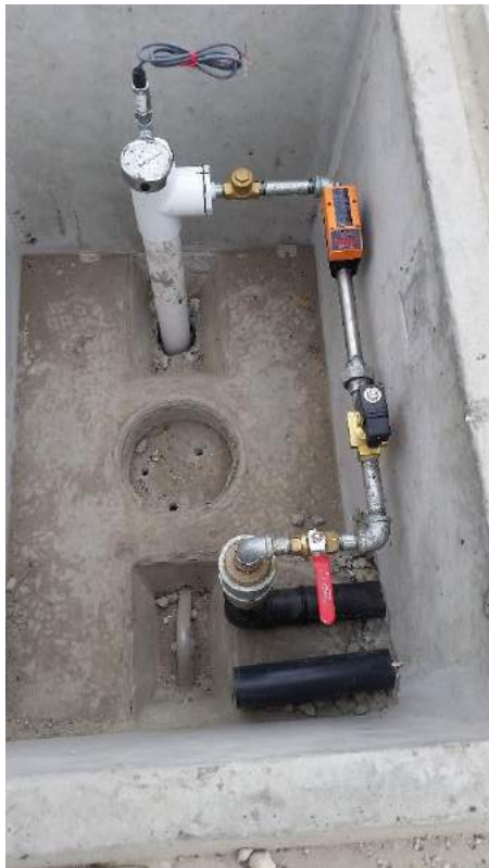
Figure 9: Well Vault Instrumentation
