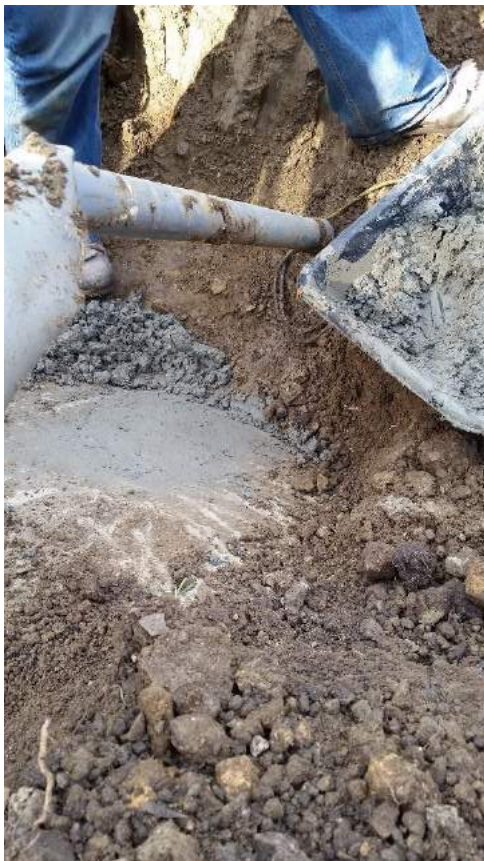
Figure 5: Plugging Storm Drain with Cement
