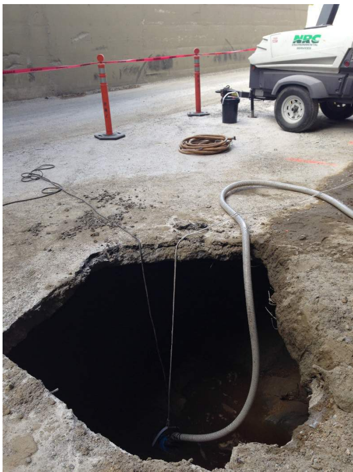
Figure 2: Ex C Pothole
