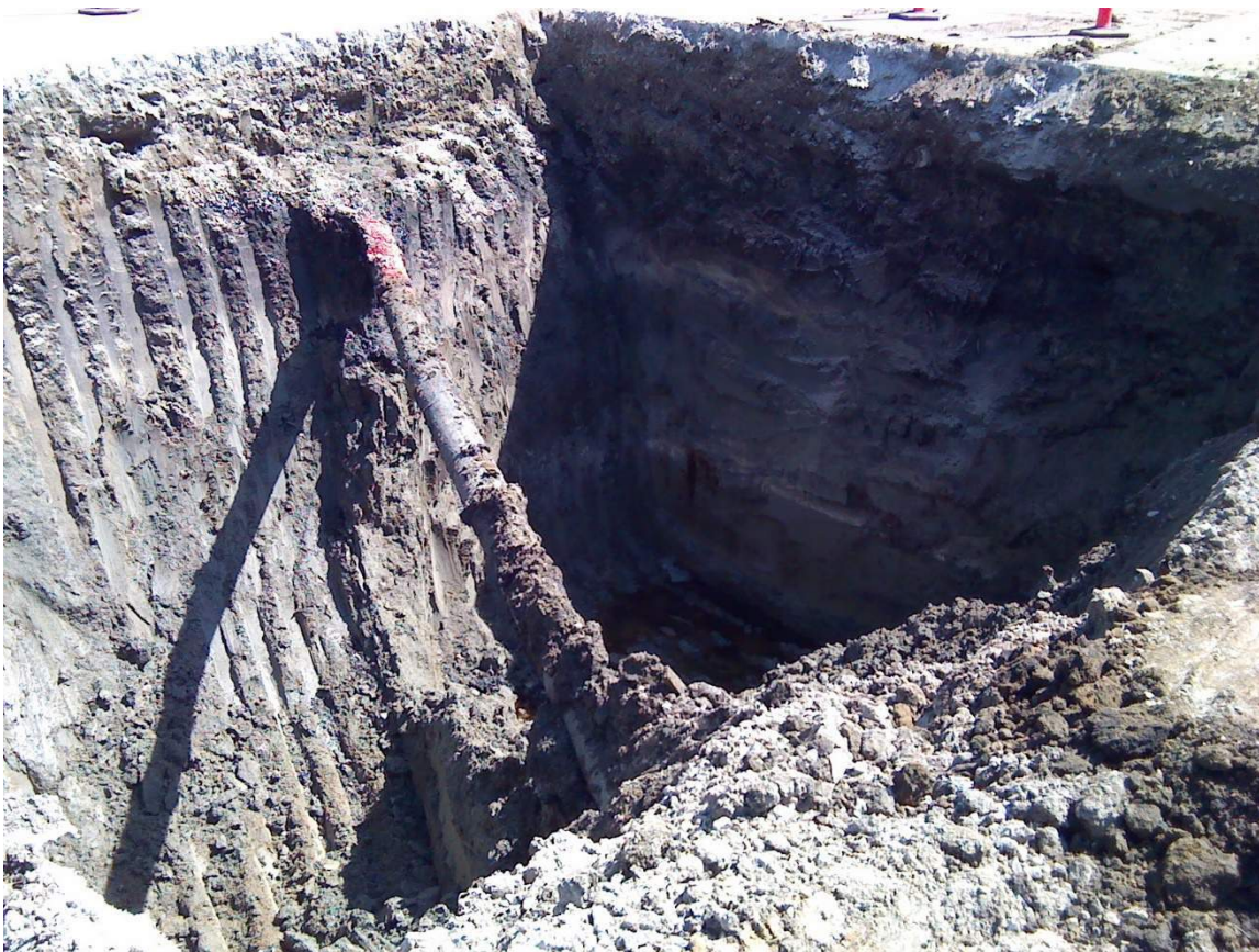
Figure 22: Exposed water pipe @ Ex E
