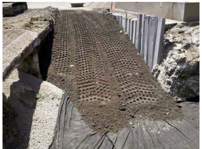
Figure 4 Clean soil placed and in the process of being compacted at Excavation D.
