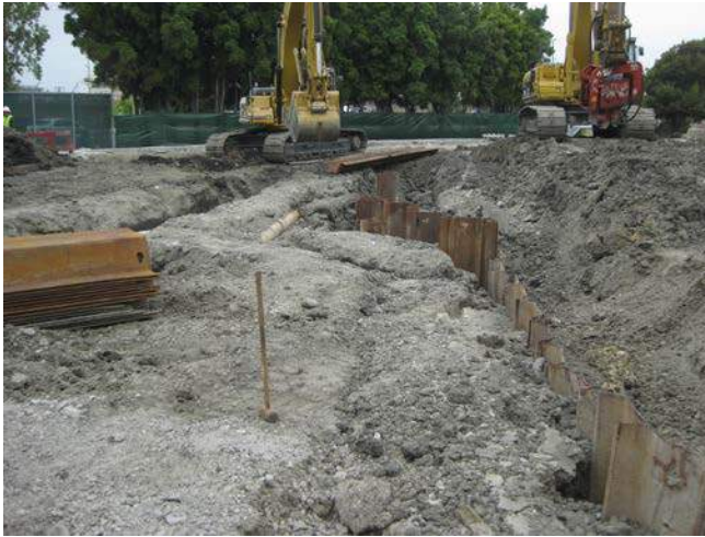
Figure 5 The trace of the active 12-inch gas line. Shoring was installed on both sides.
