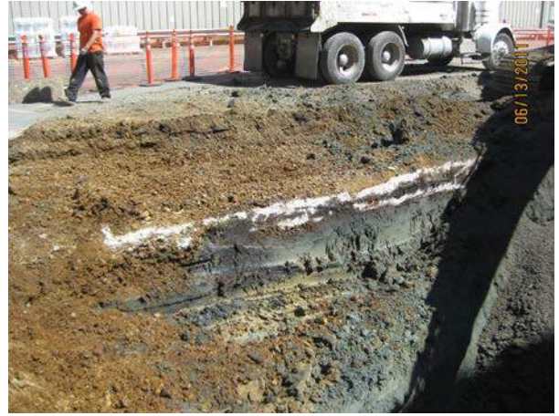
Figure 2 Looking east from the plant building at the electrical duct bank.
