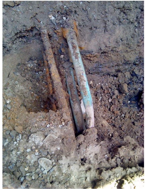
Figure 9: Dead Pipelines @ Ex C
