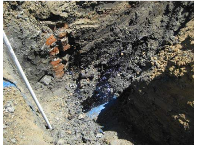
Figure 6 Part of the wall of the brick bunker visible with tar at the bottom.
