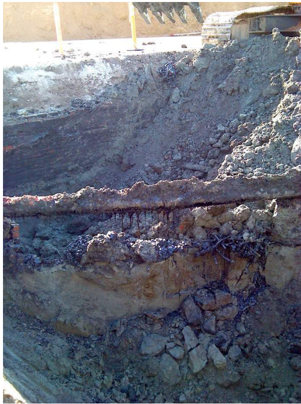
Figure 23: Tar-like Residuals on Water Pipe @ Ex E
