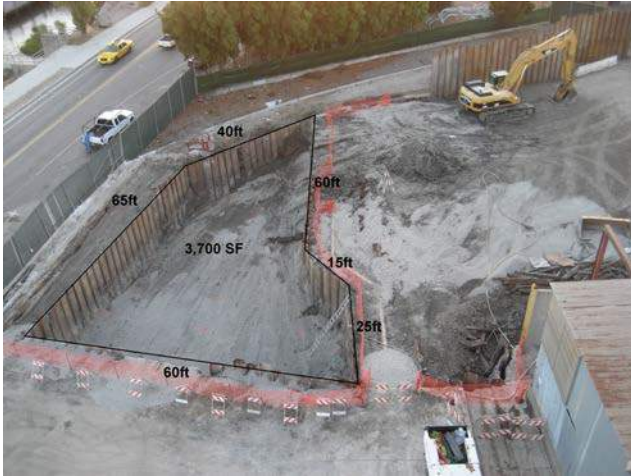
Figure 9 Aerial view of Excavation B after ORC and drain rock had been placed.
