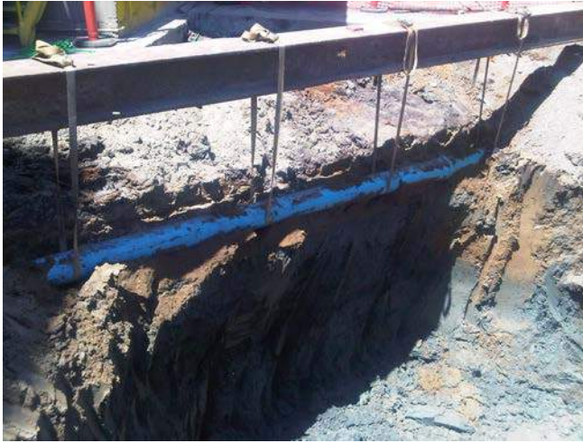
Figure 1 Northwest corner of Excavation D. The water line is supported by suspending it from an I-beam so that impacted soil beneath it could be removed
