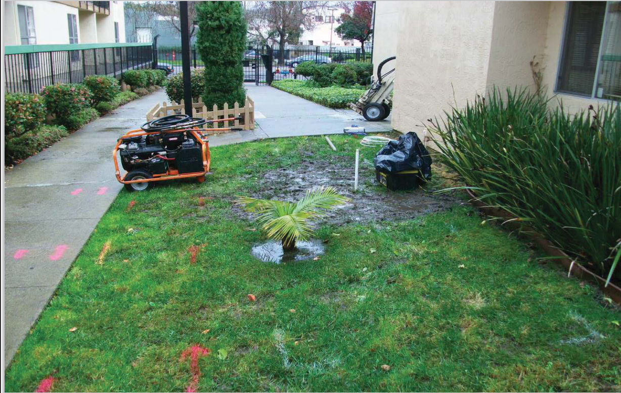
Soil boring B-4 located in the center of the subject property to the north of the leasing office structure
