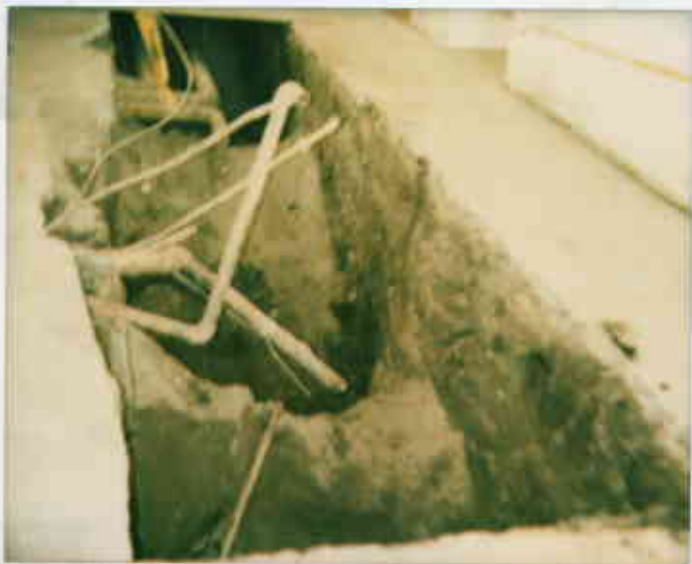
5427 Telegraph Ave. Oakland 94609 biometric pit inside the bldg at hallway (2 550G tanks removed)
