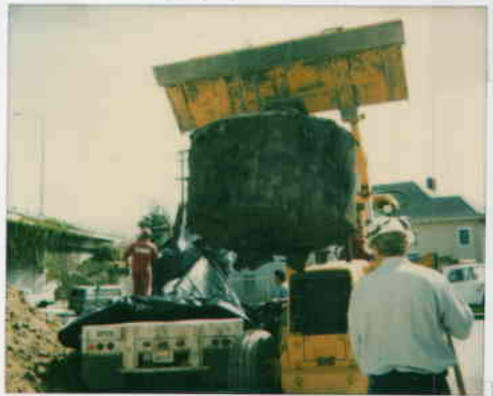
5427 Telegraph Ave. 94609 Tank #1 inside the Bldg waste oil tank. 5/11/92
