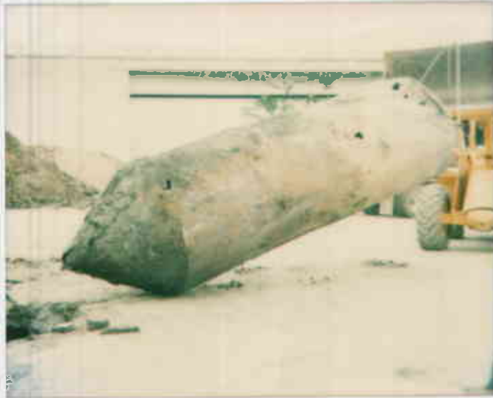
5/19/92 Tank 5427 Telegraph Ave Oakland Stoddard Tank holes 94609 at tip & sides "
