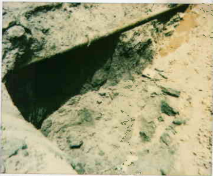
3427 Telegraph Ave 94609 Jakes Water line - Sidewalk of The Ten Tanks PT (W.A.-d)
