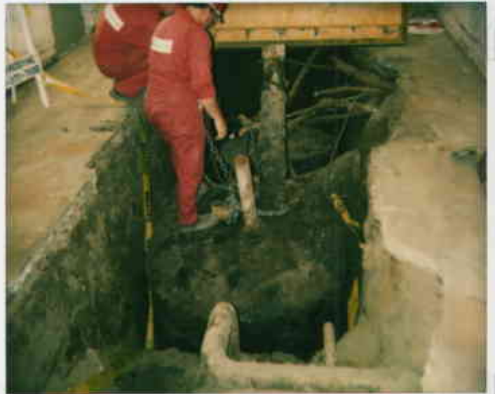
5427 Telegraph Ave. Oakland 2 tanks inside bldg 94609 in the hallway. 5/11/92
