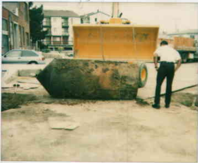
5427 Telegraph Ave. Oakland 94609 500G waste oil tank (conical shape - flat bottoms) 5/11/92
