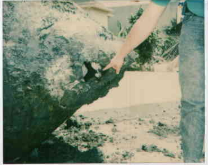
Tank II B 5-15-92 Note large hole on bottom (cono) end. Telegraph Business Park, 5427 Telegraph Av., Oak 94609 GE
