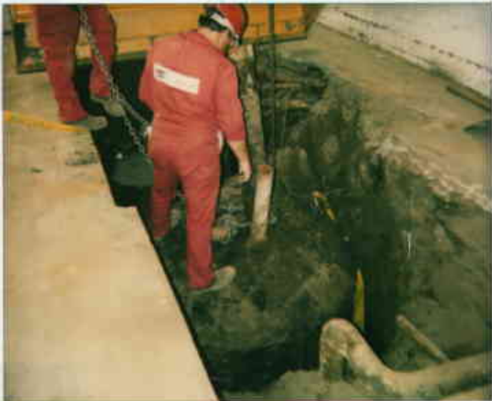
5427 Telegraph Ave. Oakland 94609 2 tanks inside the bldg in the hallway. 5/11/92
