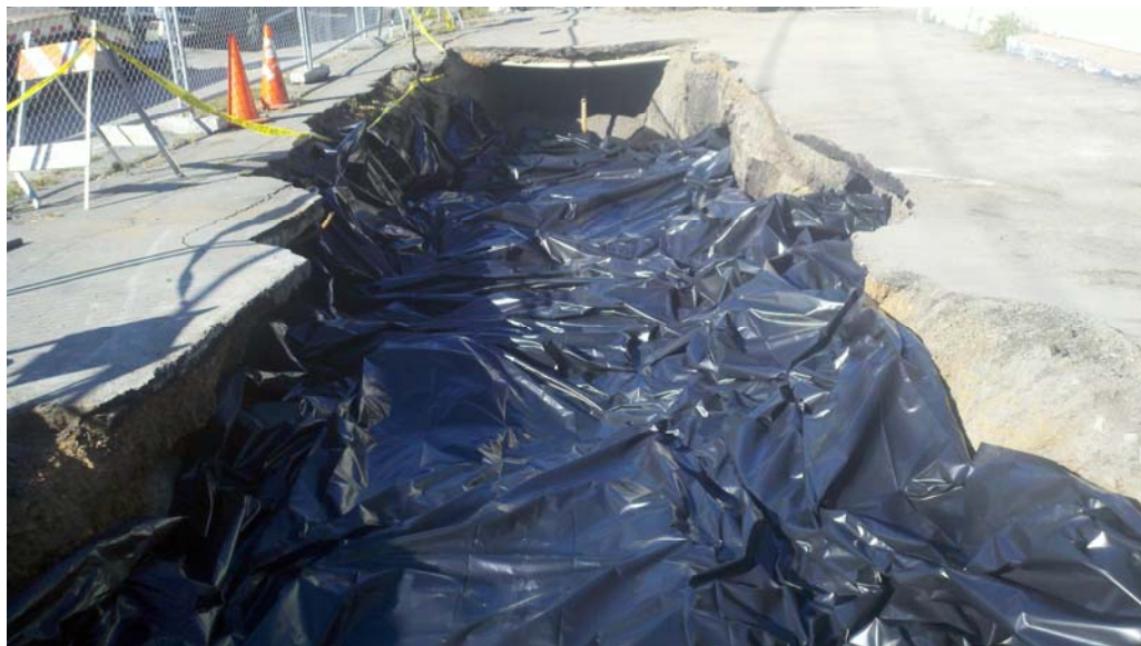
Plate 16. Layering the top of excavation with visqueen upon soil return to the pit
