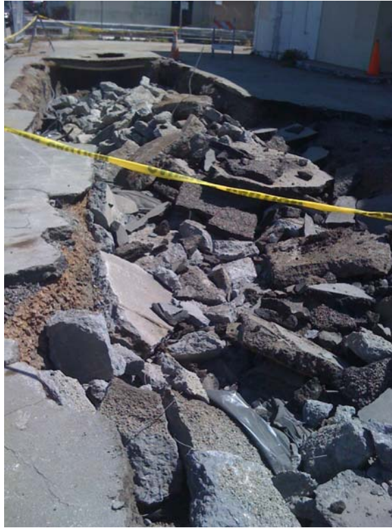
Plate 17. Concrete rubble covering the top visqueen layer
