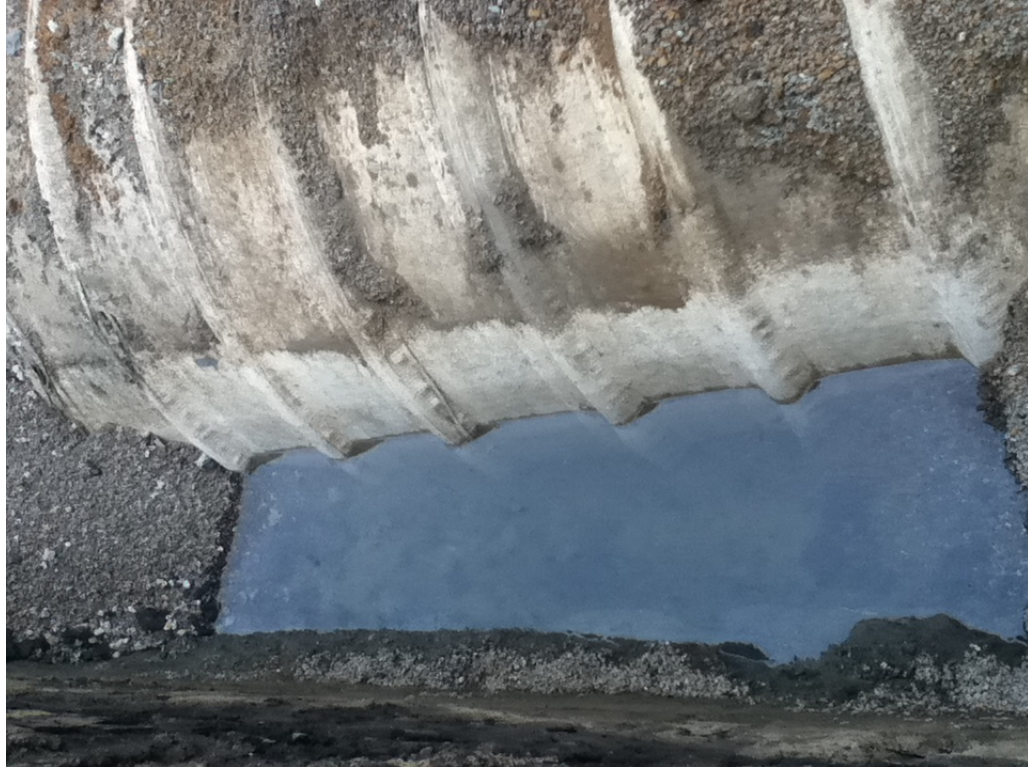
Plate 8. Standing water inside the excavation
