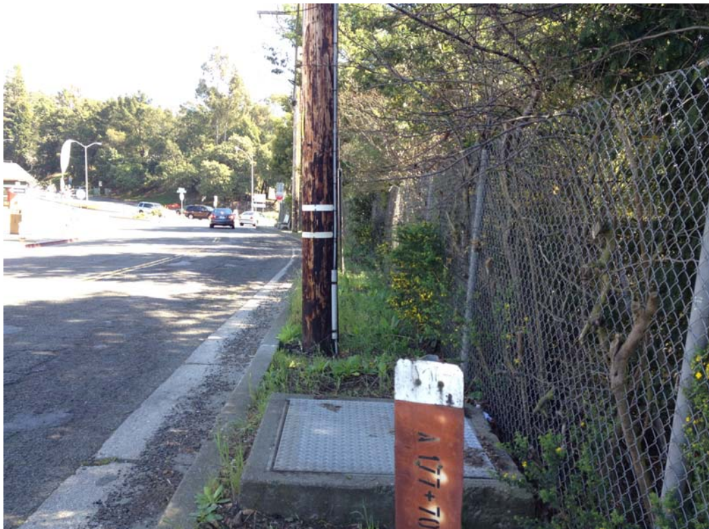
Plate 8. View of storm water manhole dirt shoulder area on Mountain Blvd.
