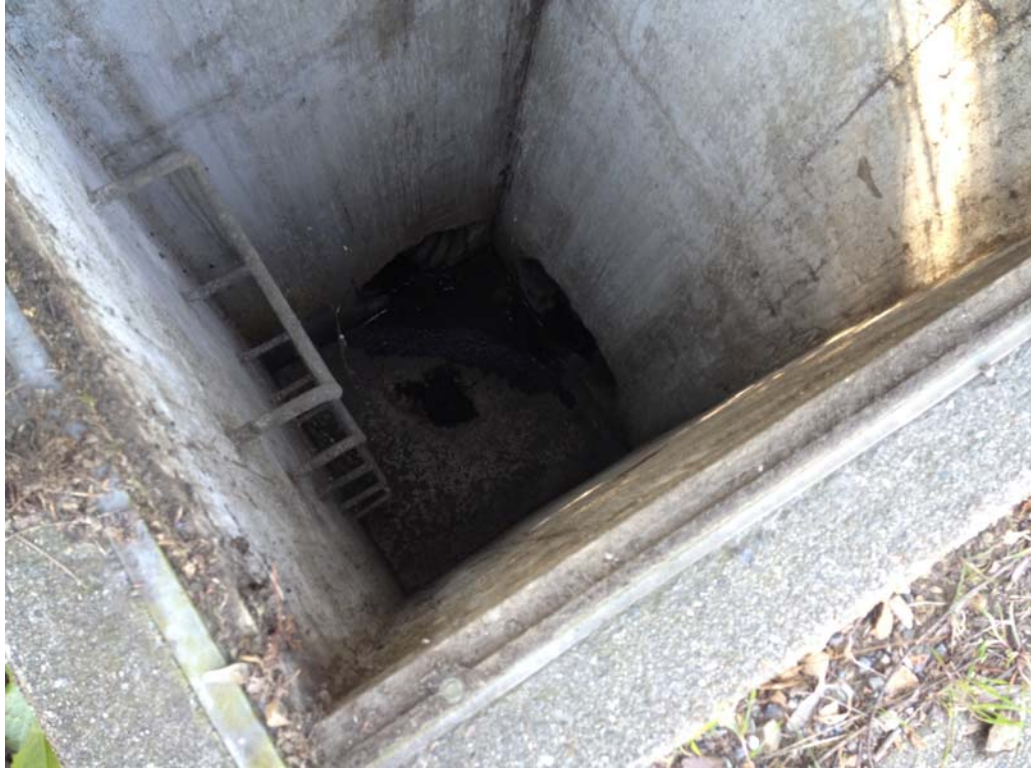
Plate 9. Inside view of storm water manhole dirt shoulder area on Mountain Blvd; no flowing water was visible
