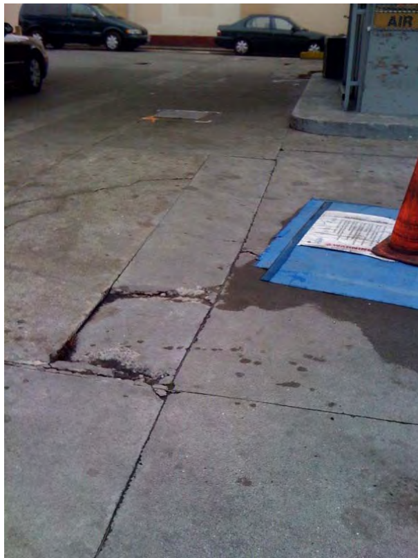
Plate 52. View of cracked / sunken concrete above former SVE trench
