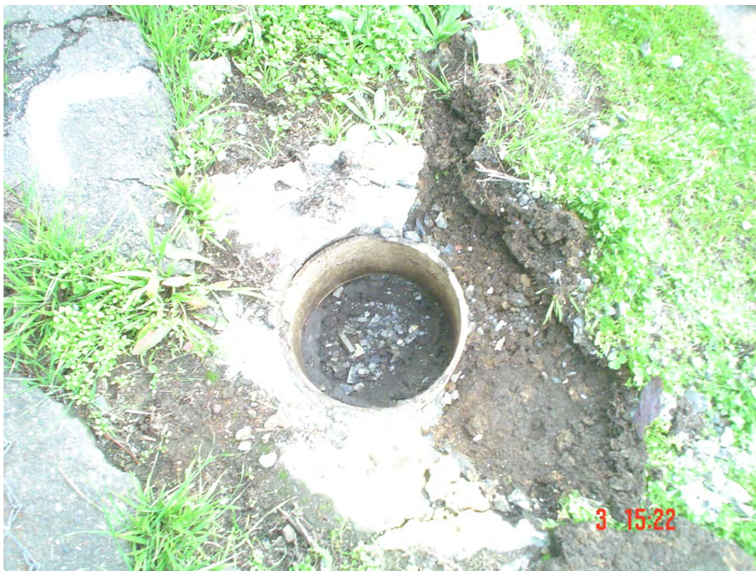
Plate 20. View of MW-10 after removing tremie grouting and removing top of casing
