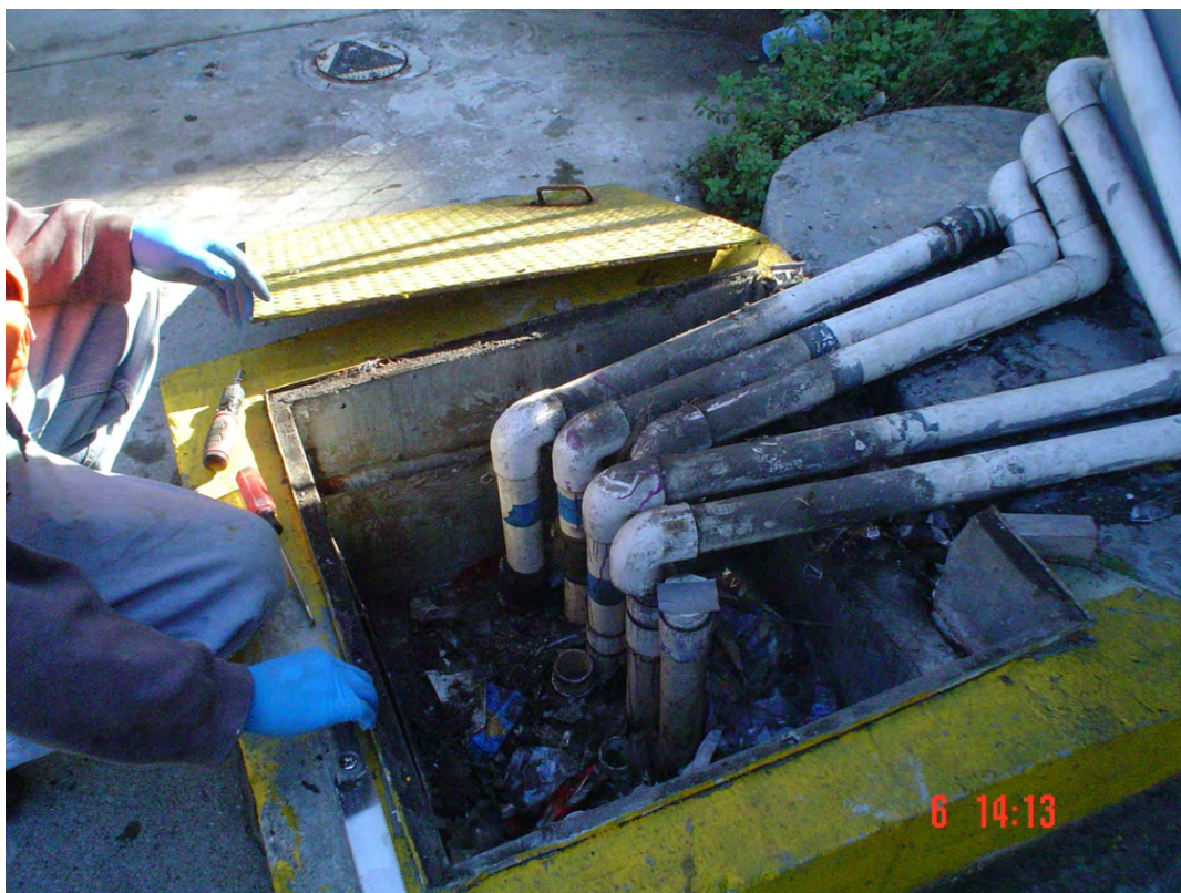
Plate 45. View of SVE and AS manifolds prior to SOMA removing piping
