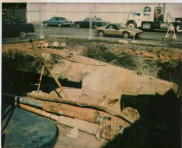
7/11/93 exposed 10k + 6k gas tanks @ Tony's Exp. Auto Serv
