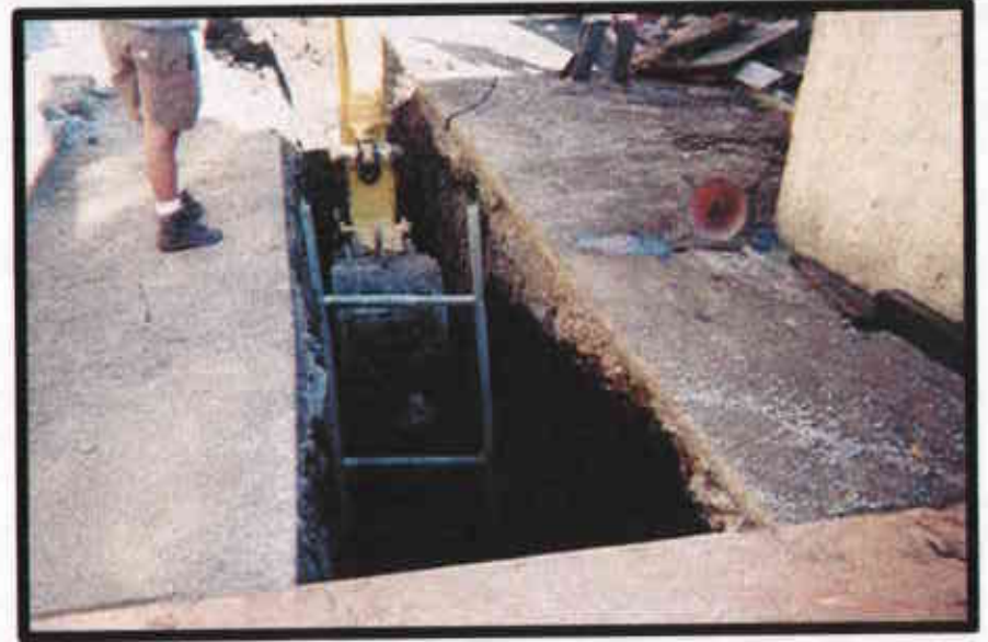
A-5: Excavating Soil After Cave-In
