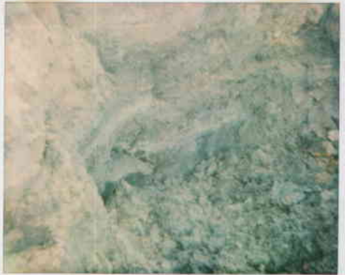
West wall B65 where brown liquid accumulates & flows Cal Trans 9/22/94
