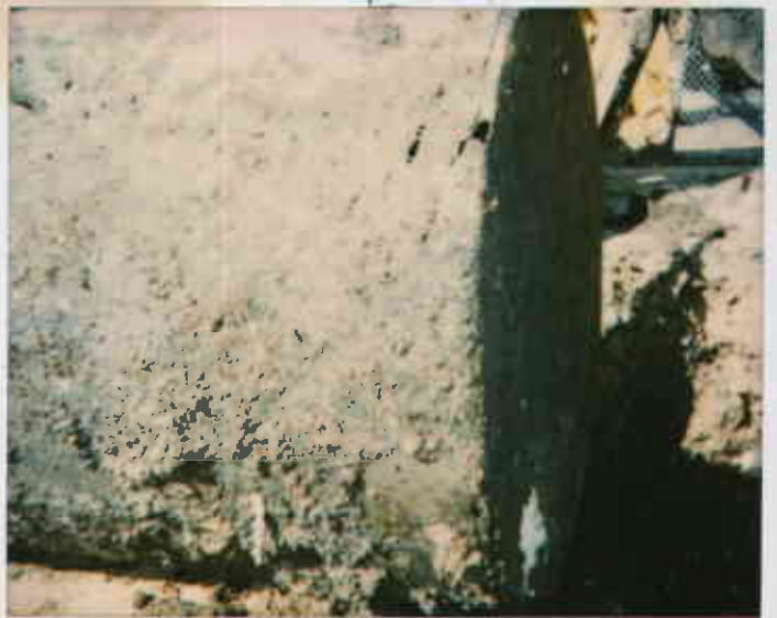
North end of Tank #4 - CalTrane holes also noted on South end 9/22/94
