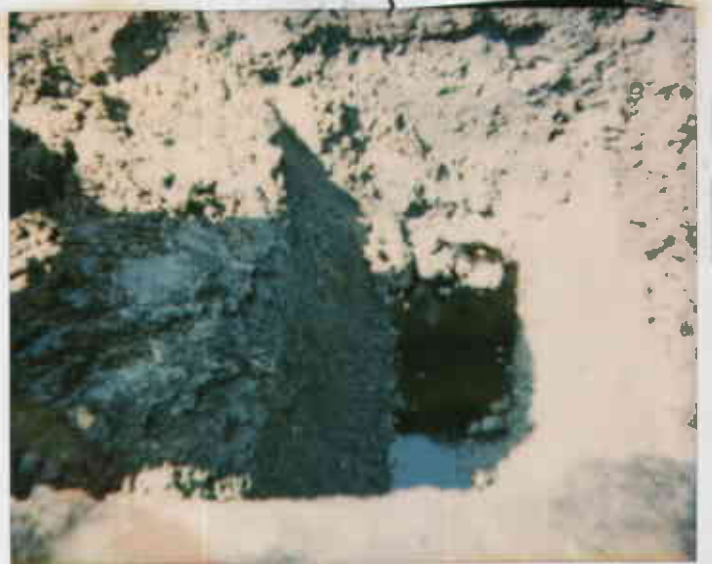
Black hydrocarbon on water beneath Tank #3 Cal Trans SSS Heyked 9/22/94
