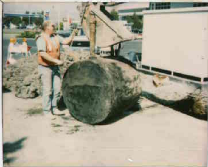
9/21/94 200 gal waste oil tank 449 Hwy Rd approx 4' wide + 4' long
