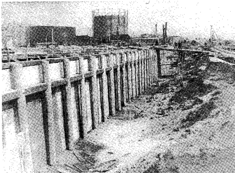
1. View of quay wall (1910-14) under construction, looking east from vicinity of Market Street, c. 1911.
