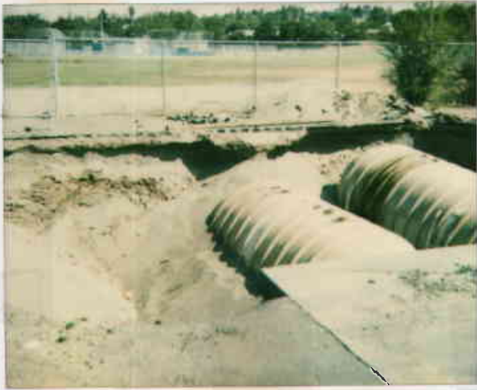
305T pit - left one broken lead in '90 Fiberglass 03216211255-8 8/6/92 ↑
