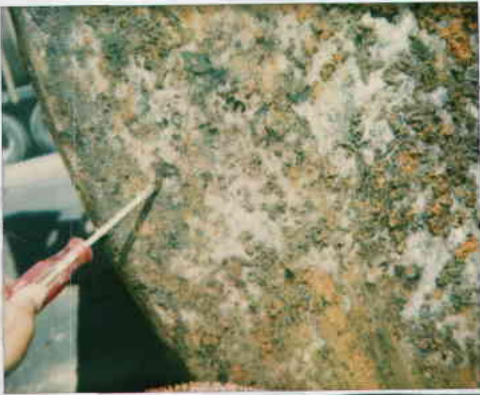
2801 Ladd 03216211255-8 8/6/92 Pin hole at fall end 2k lead gas steel
