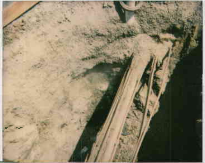
7/20/93 Photo taken by Ron Owcasz at Shell station @ 2120 Montana Ave. in Oak for piping of UGT med. where soil contamination was found at pit overexcavation. @
