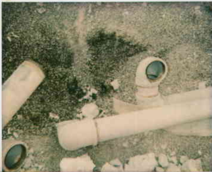
7/6/93 - Photo taken by Ron Cuccare at Banzal Shell, 2120 Hartana Ave, Oak. Shown is soil sample location at end of old pipe line for UST med. ②
