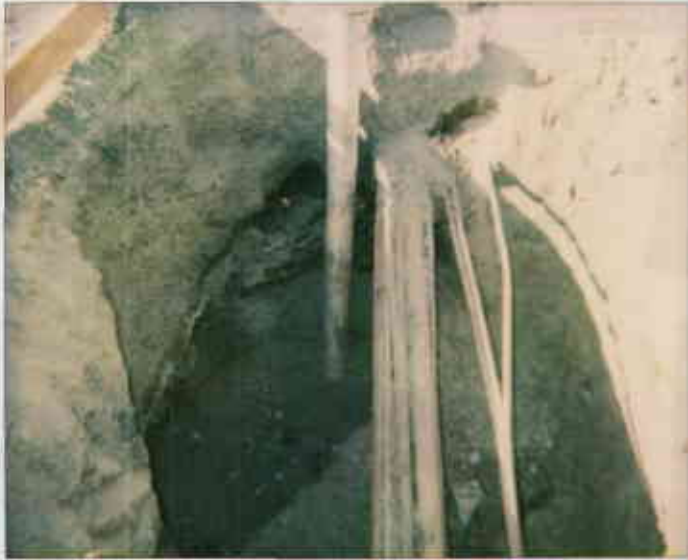
7/20/93-Photo taken by Ron Owcasz at Bansal Shell, 2120 Montana Ave. in Oak. Red caps indicate soil sample locations in side wall of pit overexcavation for UGT pipe med. @
