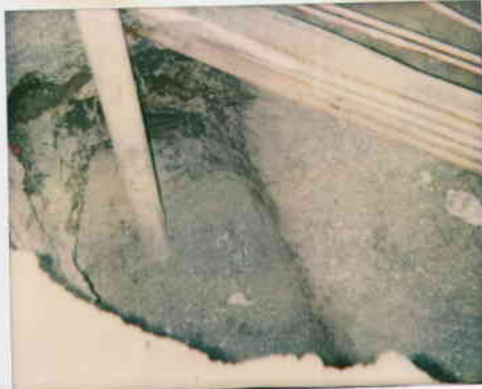
7/20/93-Photo taken by Ron Owcasz at Bansal Shell, 2120 Montana Ave. Oak. Shown is soil cont. at side wall of pit overexcavation for UGT pipe med. @
