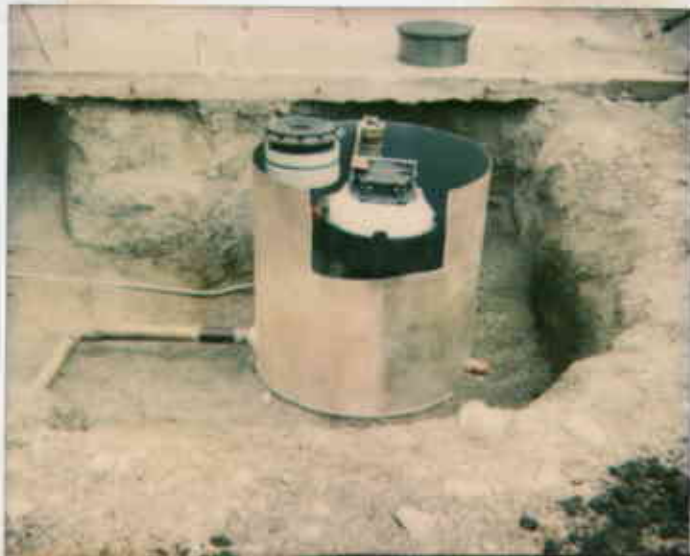
7/6/93 - Photo taken by 2215117976-B Ron Owsatz at Bansal shell, 2120 Montana Ave. Oak. Shown is new sump that failed sump test twice. Also note soil cont. at side well adjacent to it. (R)
