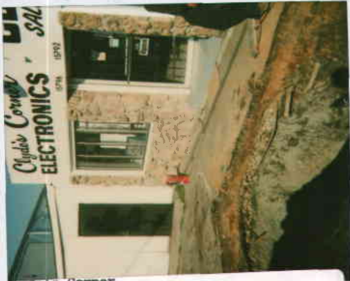
Clyde's Corner 15796 E. 14th Street San Leandro CA 94577 December 16, 1999 RW Tank Removal
