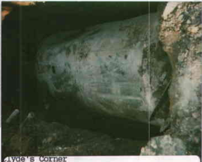
Llyde's Corner 15796 E. 14th Street San Leandro CA 94577 December 16, 1999 RW Tank Removal
