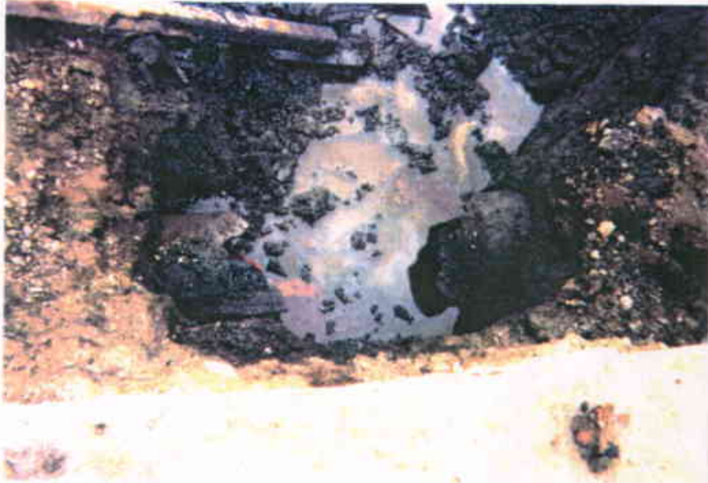
Photograph Showing Damaged Section of Lateral Loop Prepared for Repair
