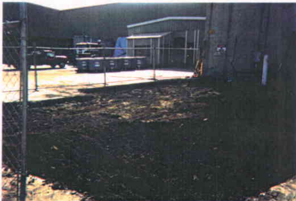
Figure 9: Photograph Looking East at Backfilled Excavation Before Final Baserock and Asphalt are Applied
