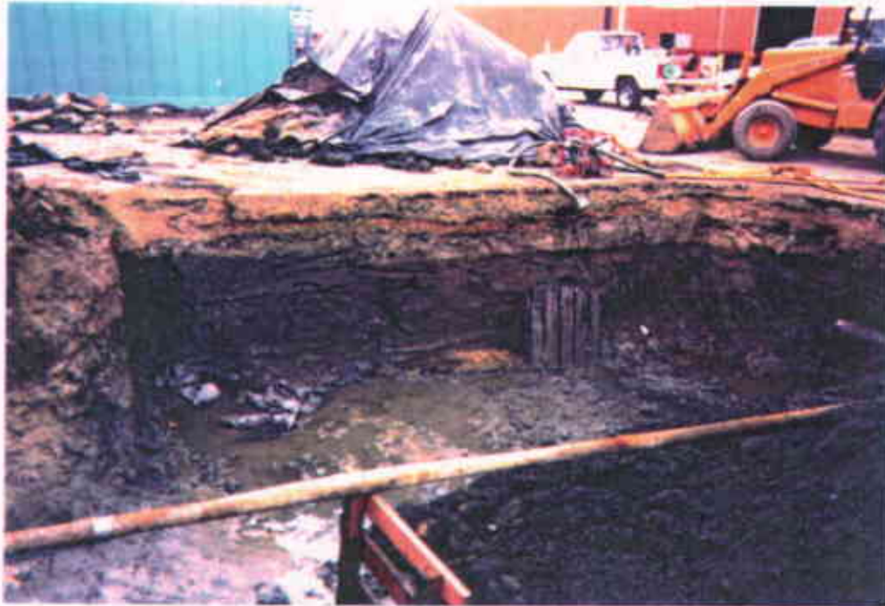
Photograph Showing West Wall of Excavation, Electrical and Telephone Conduit Spanning the Pit, and Stockpiled Soil
