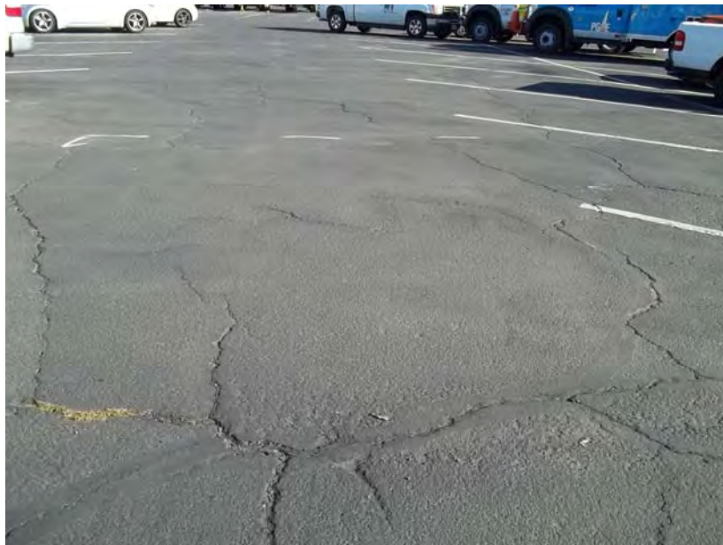
Photograph 4: Cracks in Area D
