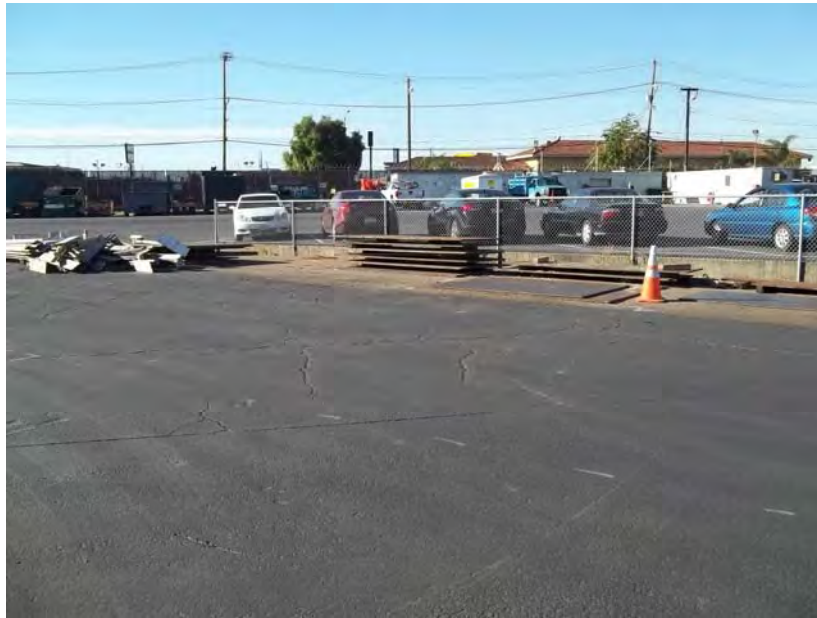
Photograph 15: Cracks in Area J
