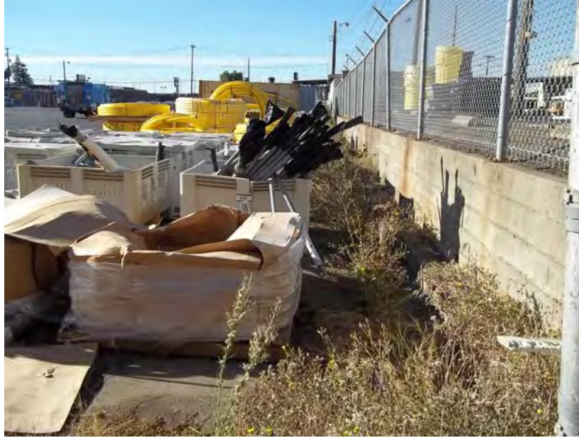
Photograph 11: Vegetation in cracks in Area G
