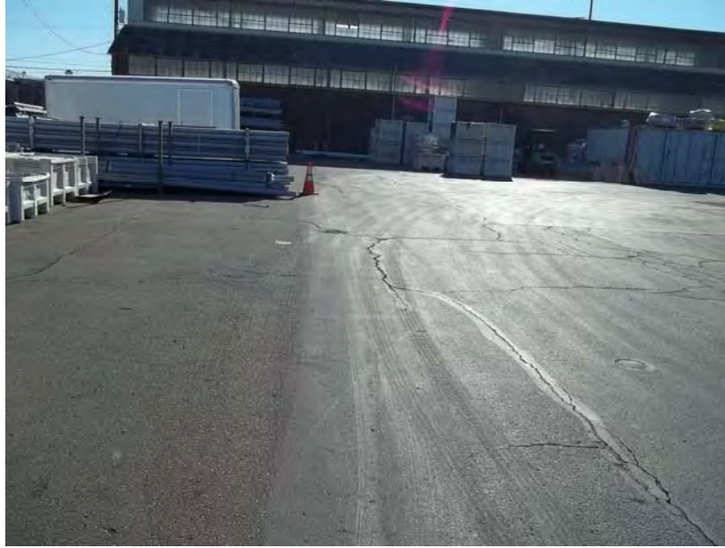
Photograph 9: Cracks in Area F
