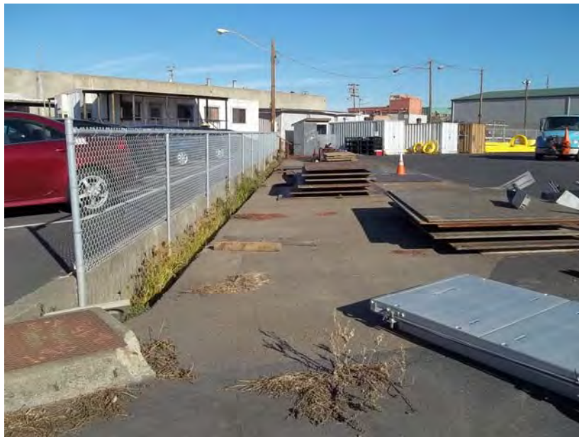
Photograph 14: Vegetation in cracks and in stormwater channel in Area K.
