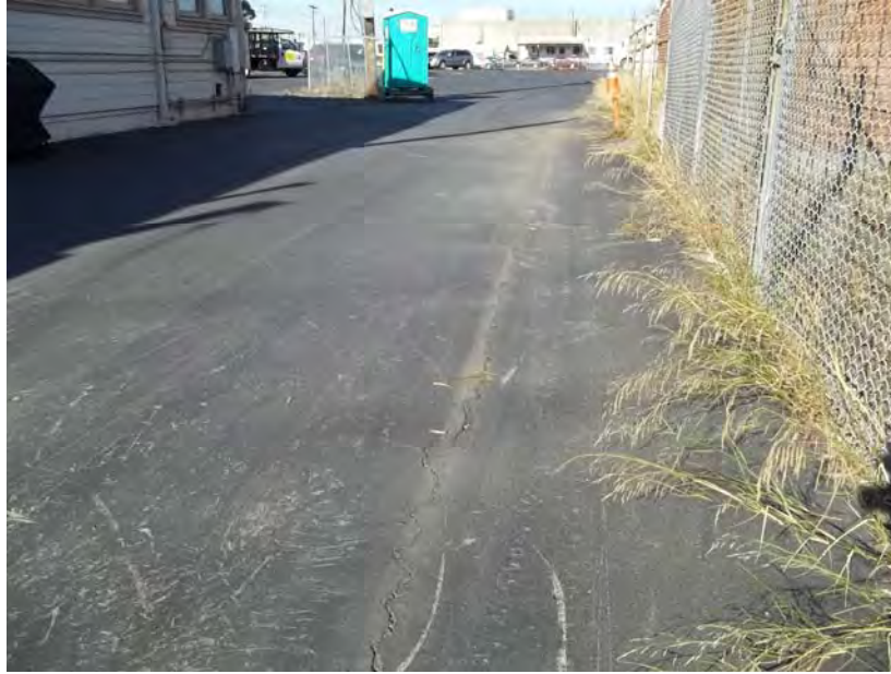
Photograph 1: Cracks in Area A
