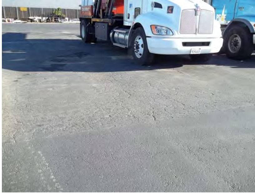
Photograph 13: Alligator cracks in Area I
