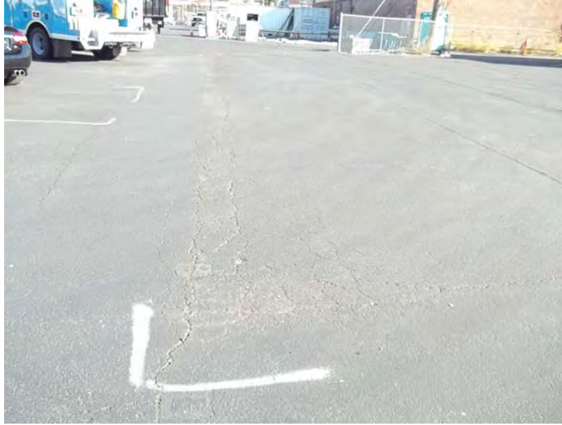
Photograph 3: Cracks in Area C
