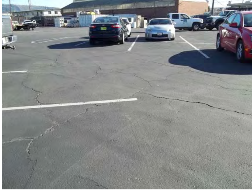
Photograph 5: Cracks in Area D
