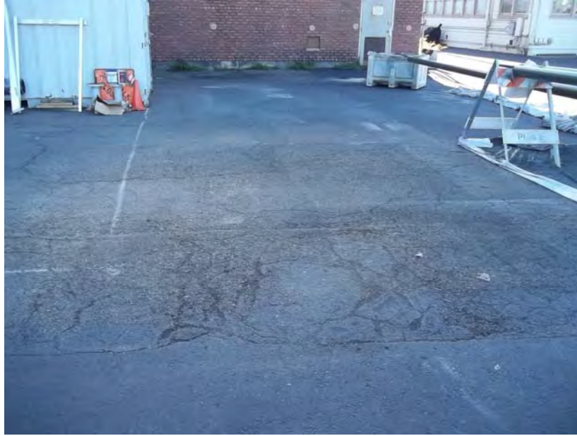
Photograph 7: Alligator cracking in Area E
