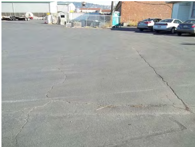
Photograph 2: Cracks in Area B
