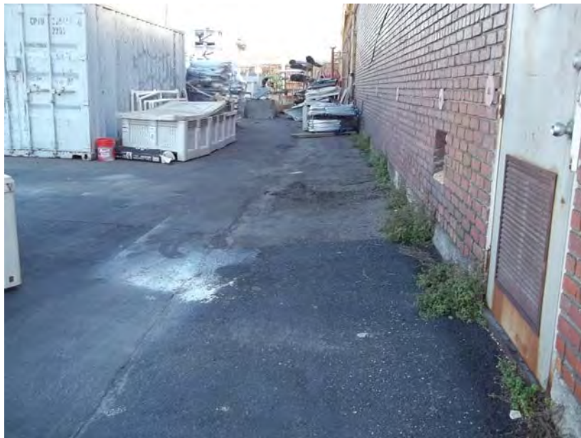
Photograph 6: Vegetation and cracks along wall of adjacent building in Area F
