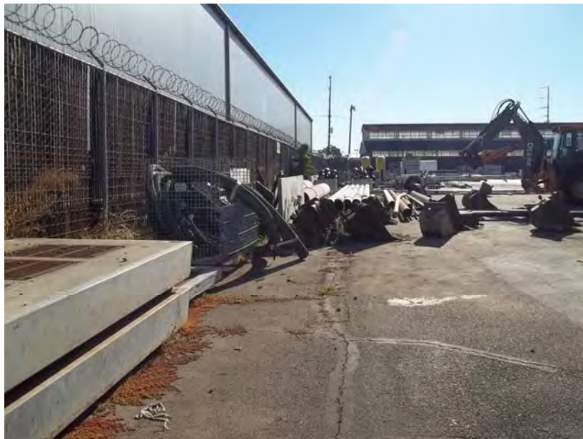
Photograph 10: Cracks in Area F, and vegetation in cracks in Area G
