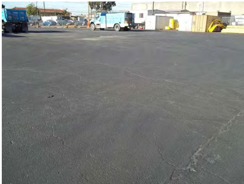
Photograph 12: Cracks in Area H
