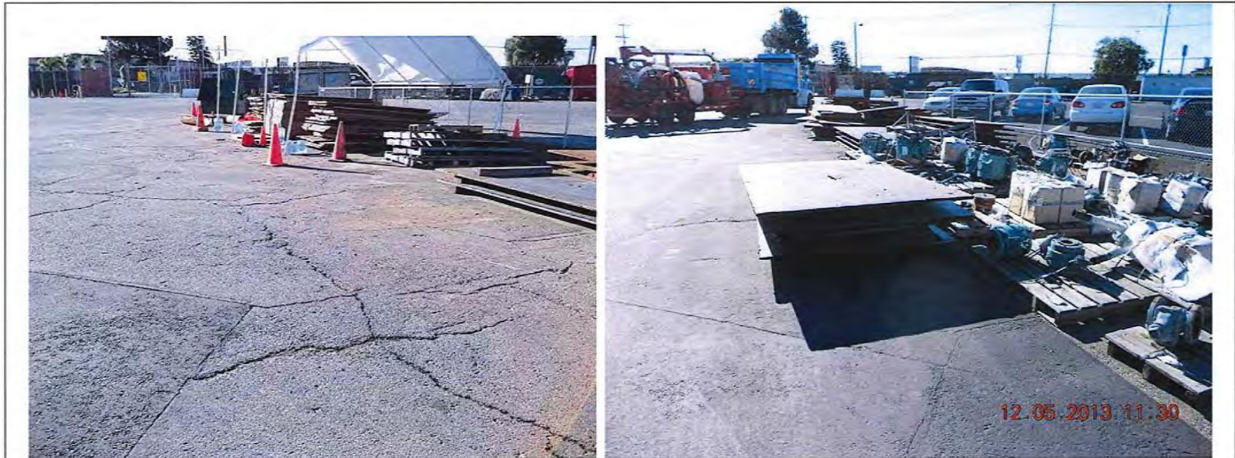
Photographs 11A and 11B: Cracking and weathered surface in Area M of the 2012 report. In 2013 some of the area has been sealed.
