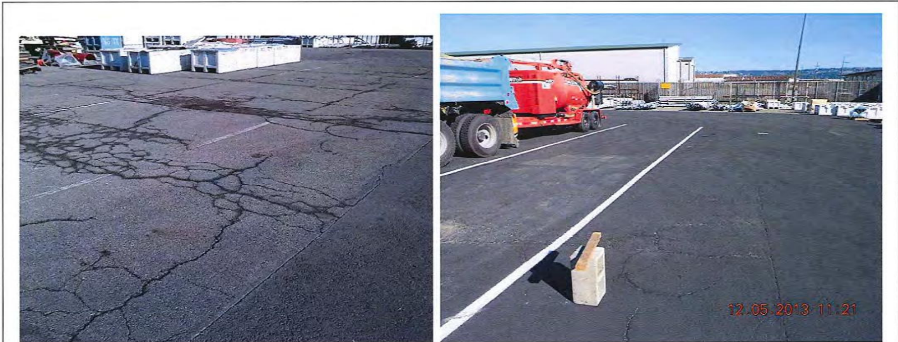
Photographs 3A and 3B: Cracking and pavement failure in Areas B and C of the 2012 report. In 2013, the area has been sealed.
