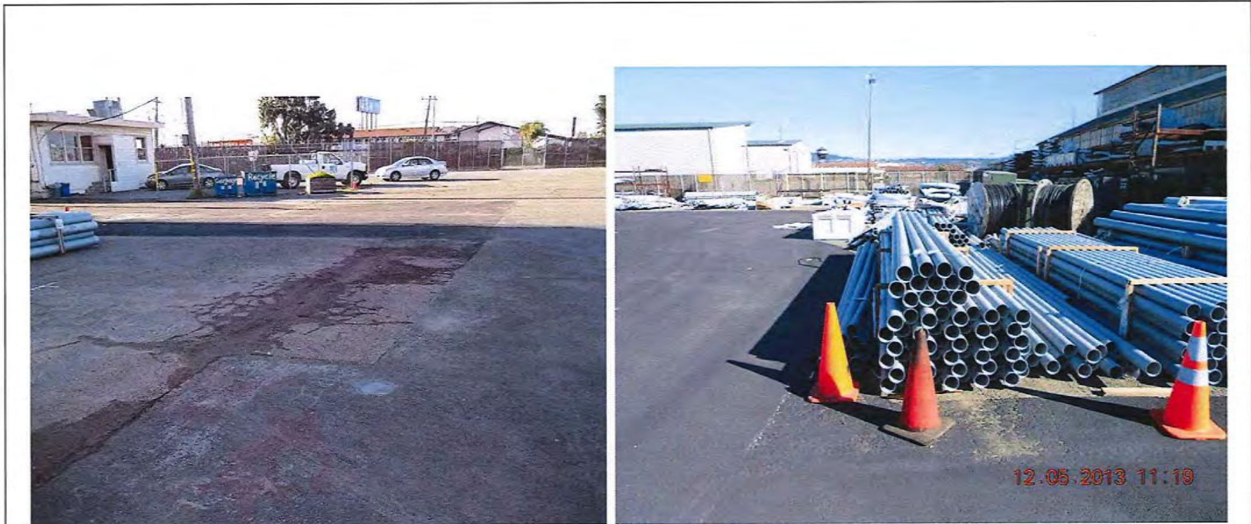
Photographs 1A and 1B: Pavement failure in Area A, 2012 on the left. The area was not visible due to materials storage in 2013 (the 2013 photo was taken facing east).
