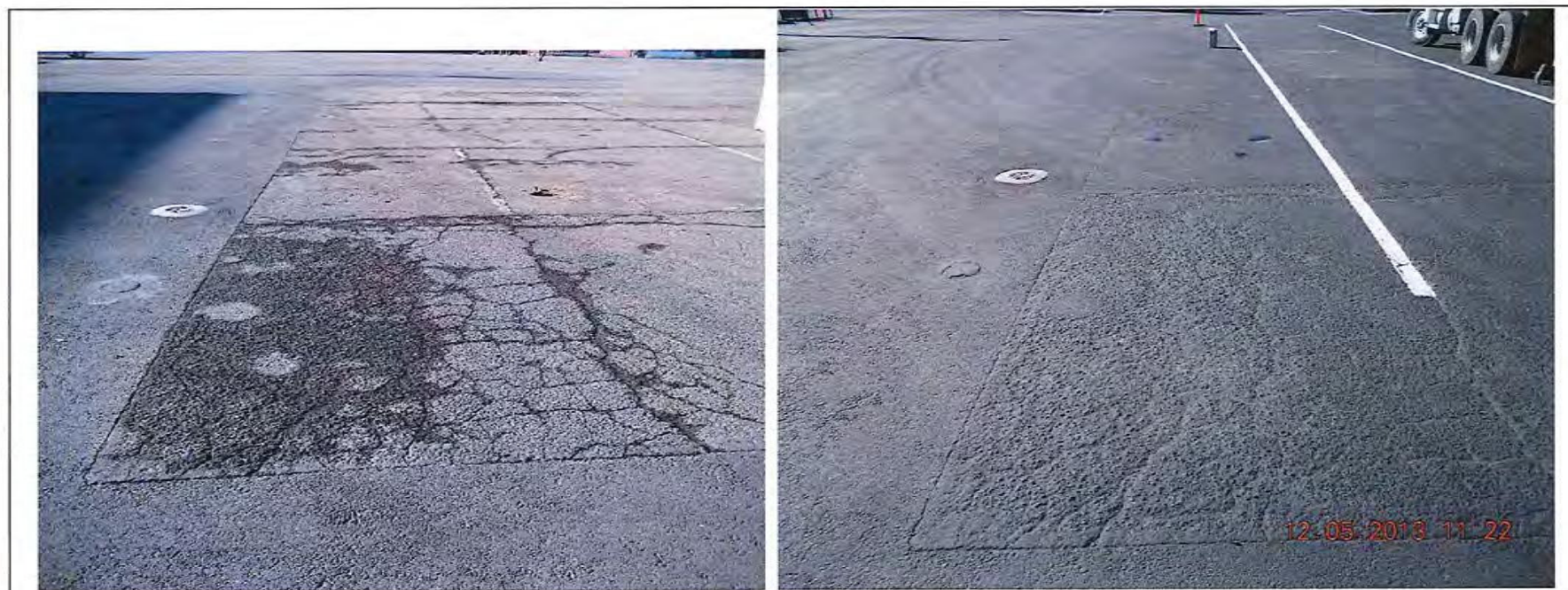
Photographs 4A and 4B: Pavement failure in Area D of the 2012 report. In 2013, the area has been sealed.
