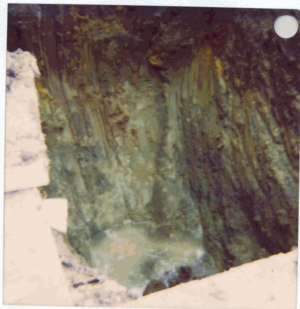
4028 E 14th St. Oakland Overexcavation down to groundwater @ 11' bgs contamination apparent on side walls
