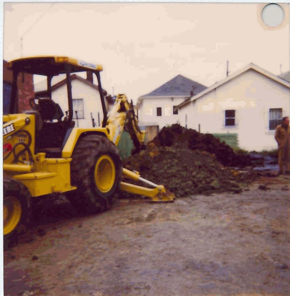
4028 E 14th St. Oakland Overexcavation of backfill & native soils w/ 18 c.y. of contaminated soil.
