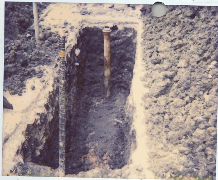
5/11/93 STID 805 Exposed tank - bigger than 5000 G
