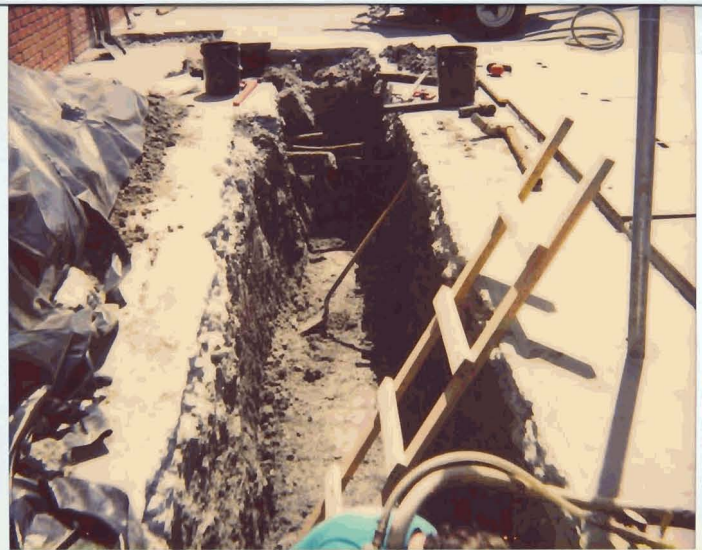
STID 805 1001 - 4and Emerysville 4400 with later lines / product lines at southern end of PIT. 5/13/93 exposed tank for (10,000 G)
