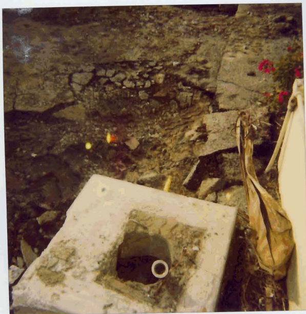
under fuel dispenser photo 3
