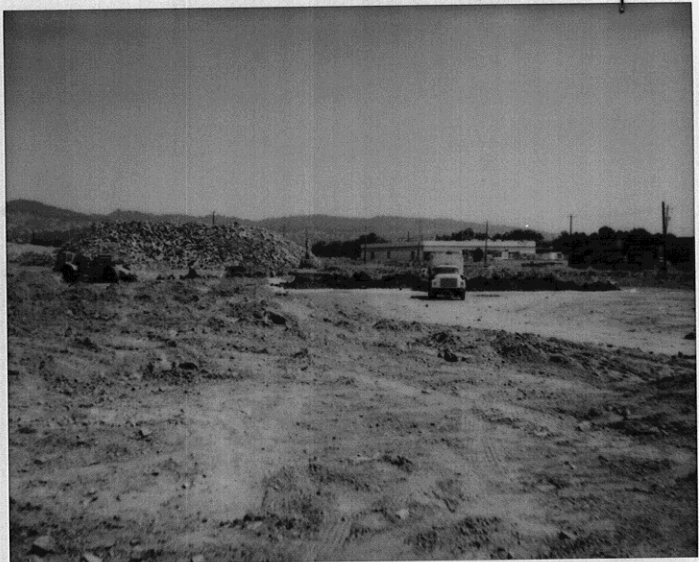
9/2/93 STID 1667 Aeration beds Yuba Bussa Project
