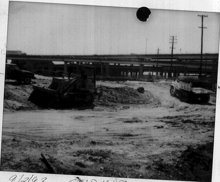
9/2/93 STID 1667 Aeration beds Yuba Bussa Project
