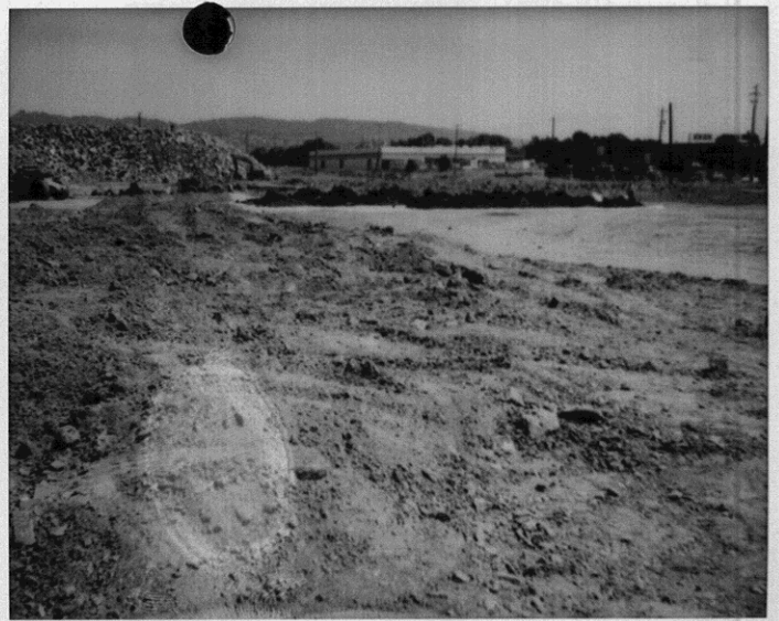
9/2/93 STID 1667 Aeration beds Yuba Bussa Project
