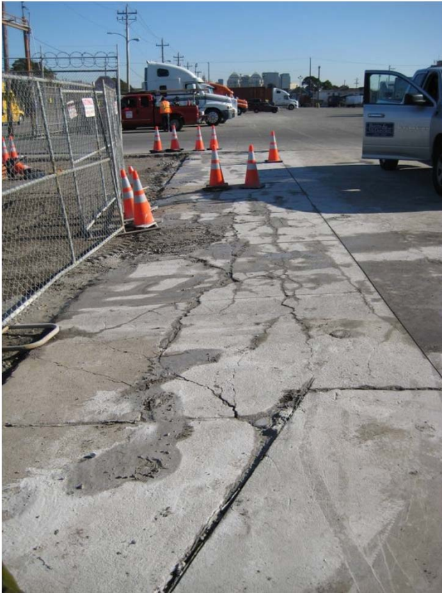
Concrete Damaged due to Weight of Excavator- South of UST Pit
