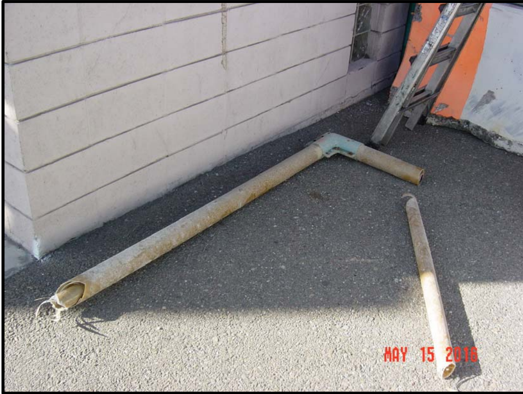
Photograph 5: Double-walled fuel conveyance pipe.
