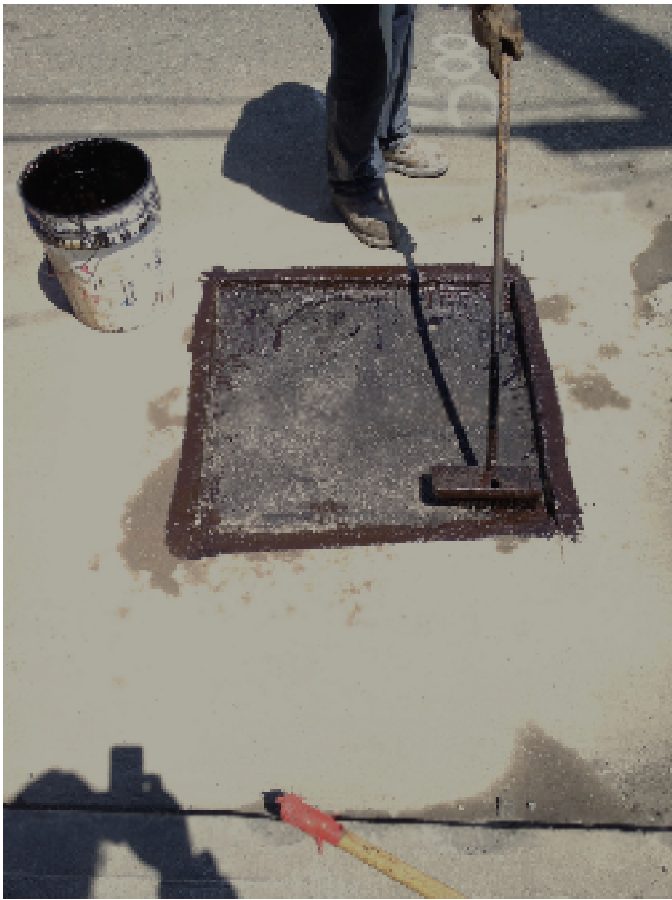
20 August 2012. View of well MW4 during repaving. The first layer of hot mix asphalt concrete has been placed and compacted. View looking northeast.
