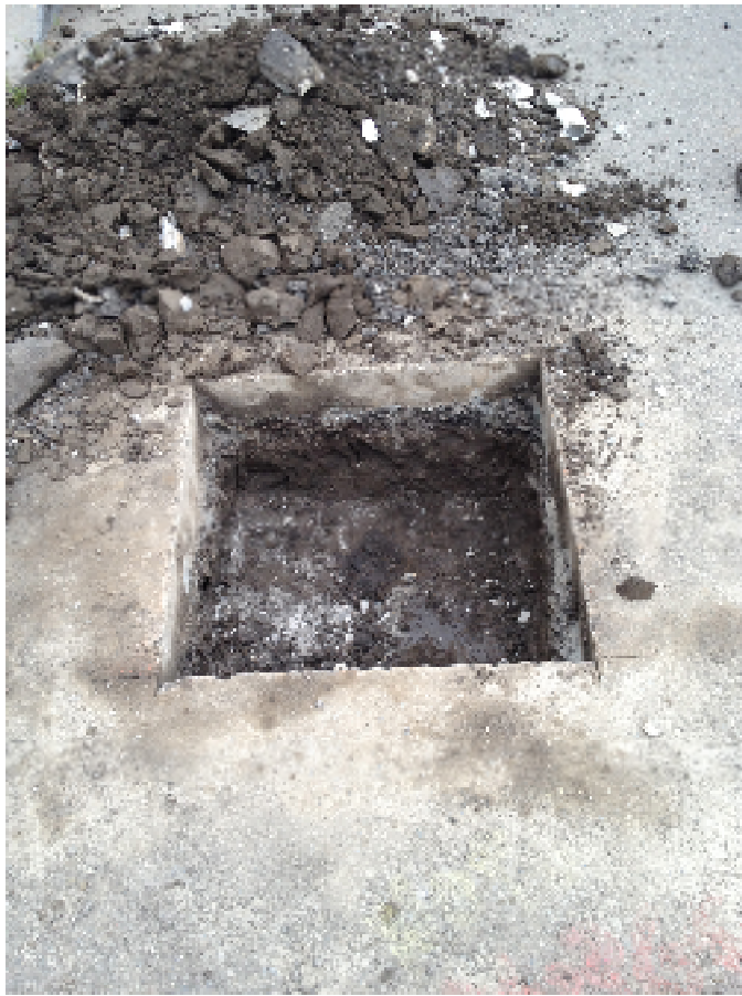
20 August 2012. View of well MW5 after grouting, overdrilling, and excavating to a depth of \pm 18 inches. View looking northwest.
