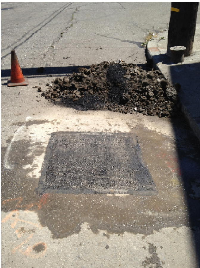
20 August 2012. View of well MW4 after repaving. The second (final) layer of hot mix asphalt concrete has been placed and compacted. View looking southeast.
