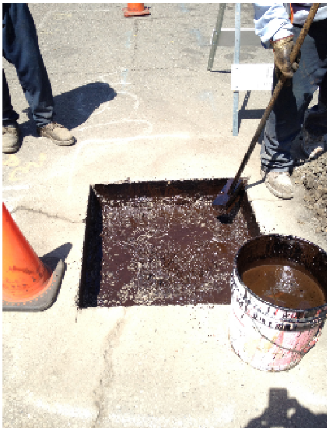
20 August 2012. View of MW5 after placing and compacting aggregate base but before placement of asphalt concrete. View of placing tack coat. View looking southeast.
