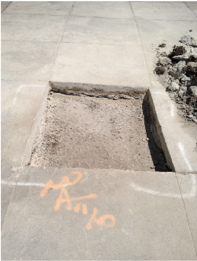
20 August 2012. View of well MW1. Aggregate base has been placed and compacted. View looking northeast.
