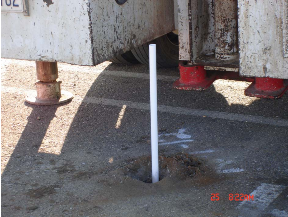
Photo #7 - Temporary piezometer with 3/4-inch diameter PVC screen and riser pipe being installed in borehole RM-12.
