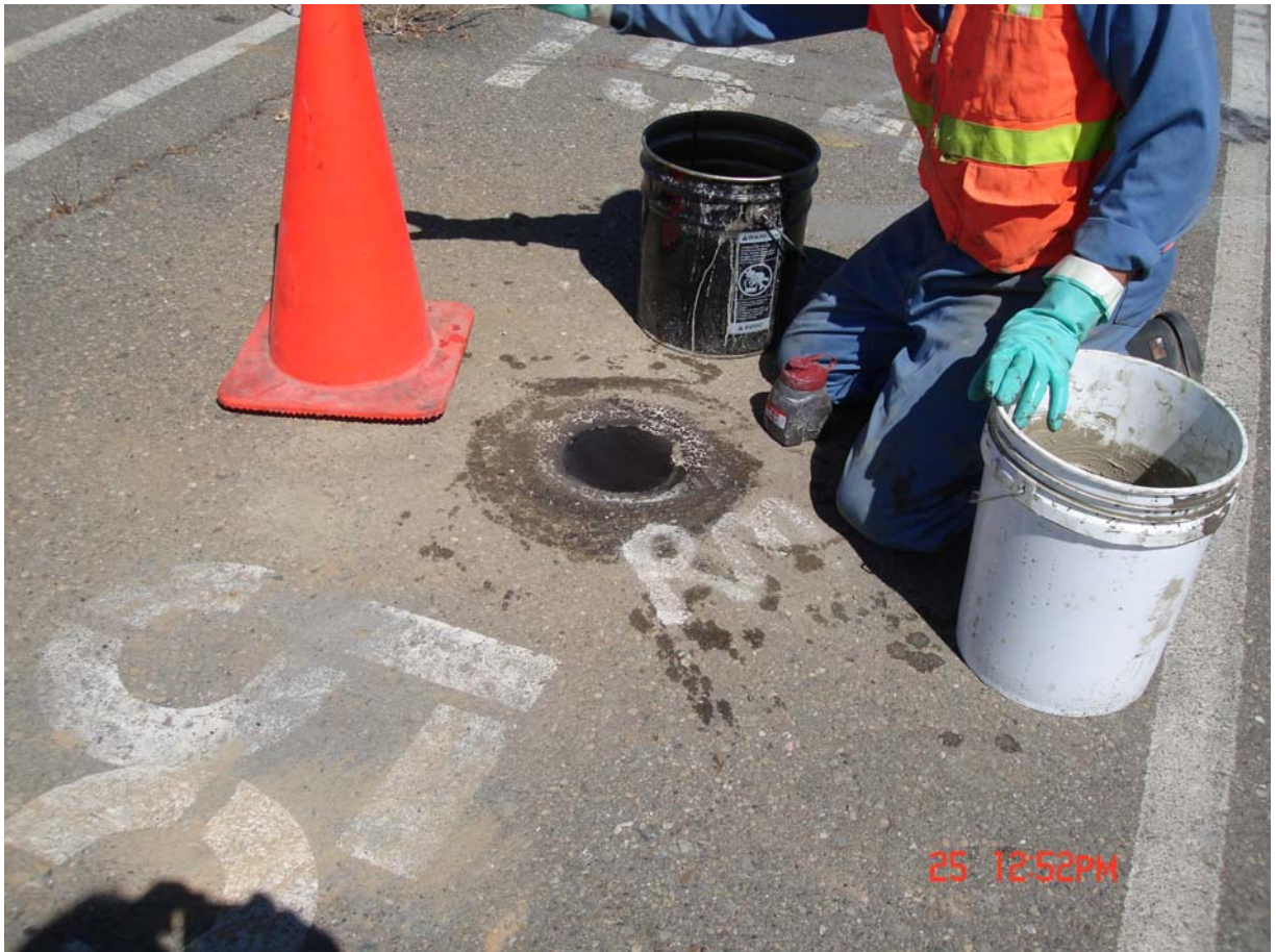
Photo #8 - Borehole being topped off with cement slurry and dyed to match the surrounding surface.
