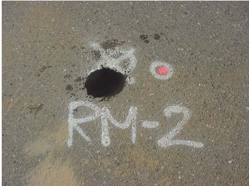
Photo #10b (3/15/07) - Completed surface finish of boring RM-2, note the color of the dyed concrete cap
