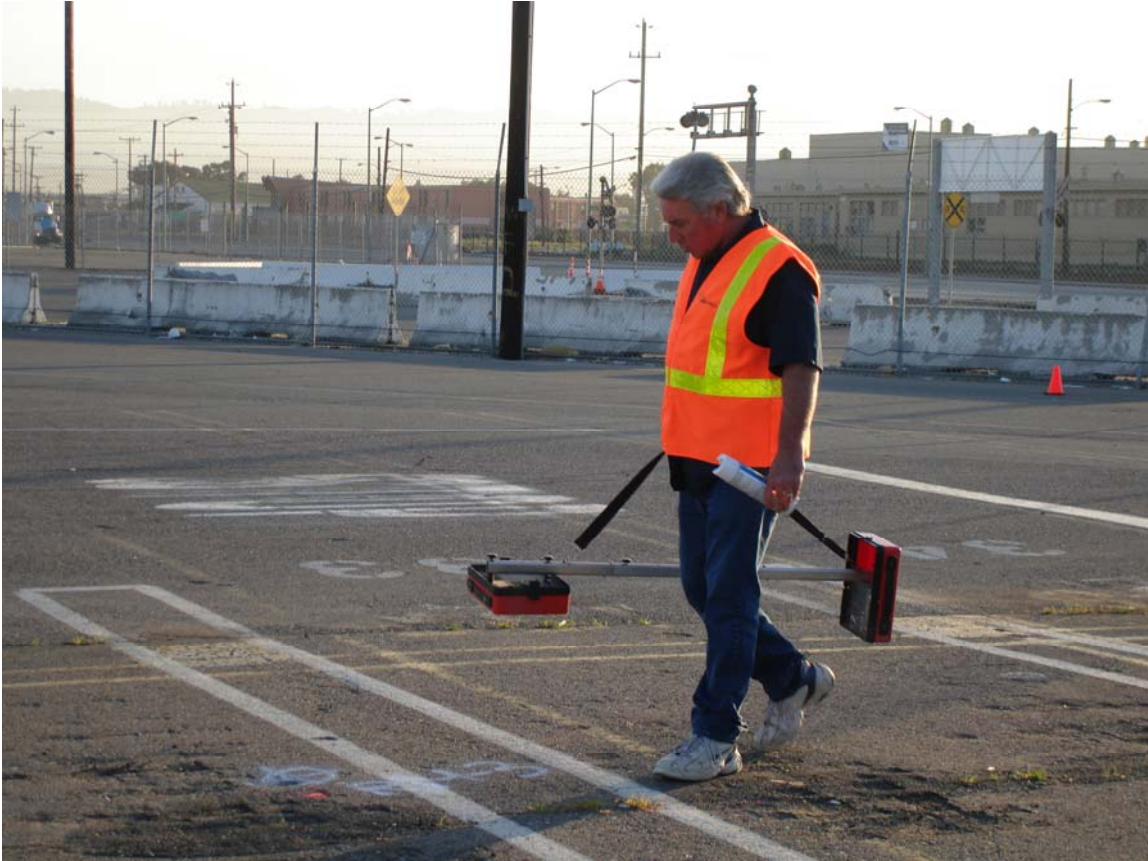
Photo #3 (3/13/07) - Subsurface utility locator clearing proposed borehole locations of subsurface piping with metal detector
