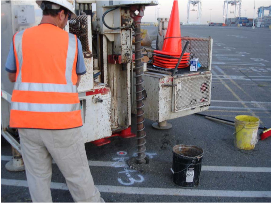
Photo #4 (3/15/07) - Driller using hollow-stem auger to break through pavement prior to hand auguring to 5 ft in RM-3
