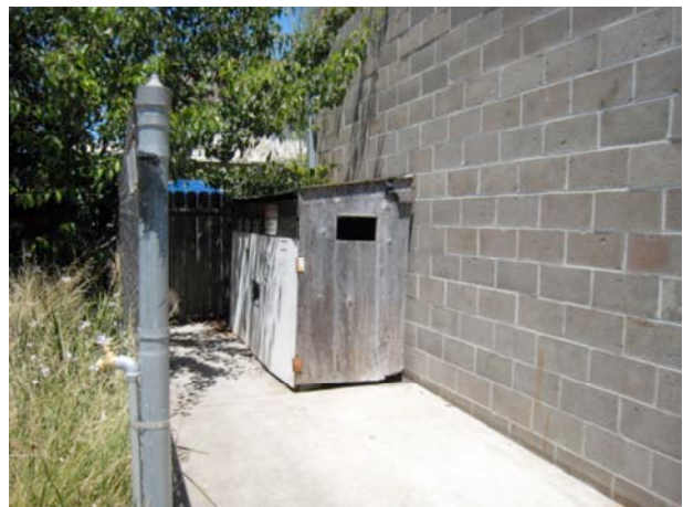
28. View of the storage shed located near the southwest-facing elevation of the paint shop.
