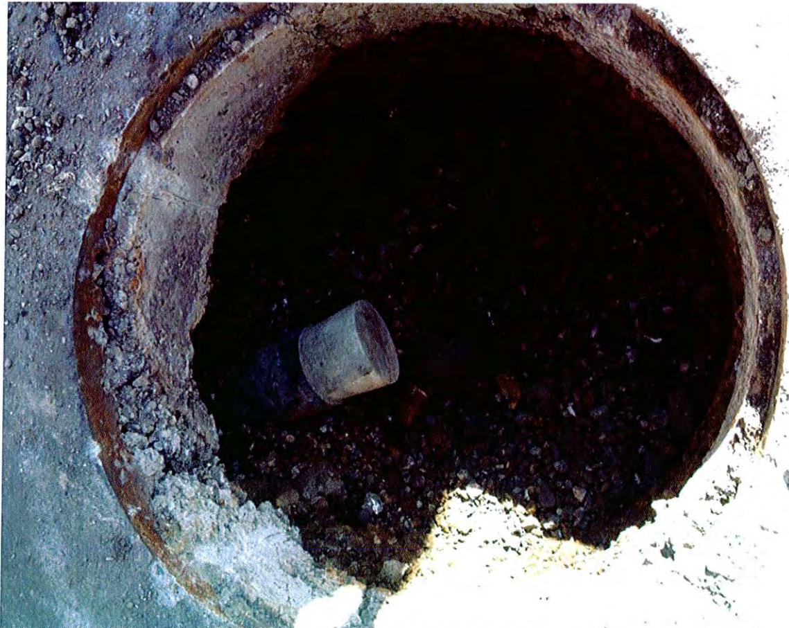
MW-4 – Capped Conveyance Line
